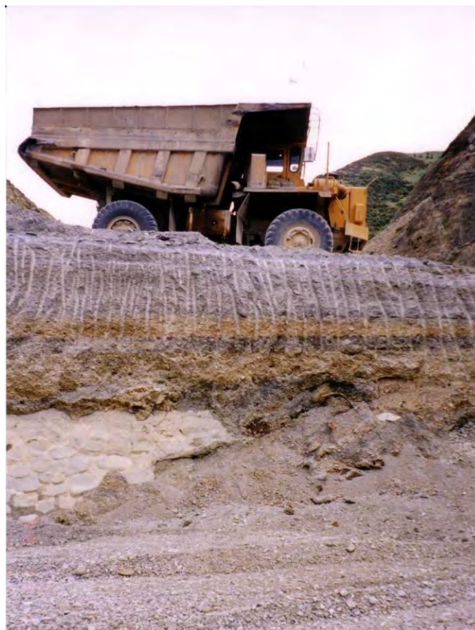
Dumper moving along old coastal road area shows the extent of fill above the old rock wall.
