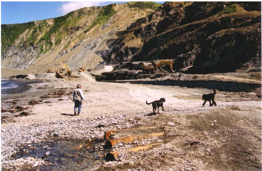
Hape Stream mouth work nearing completion. Digger placing riprap along exposed concrete road. Exposed rock wall in foreground.
