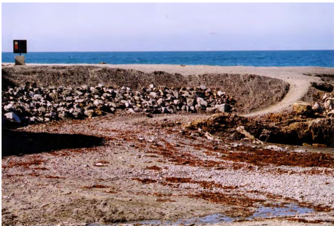
After removal of stockpiles and concrete, the area starts to take shape.
