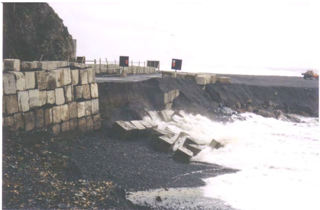
Sea wall collapsing into the sea during a southerly storm.
