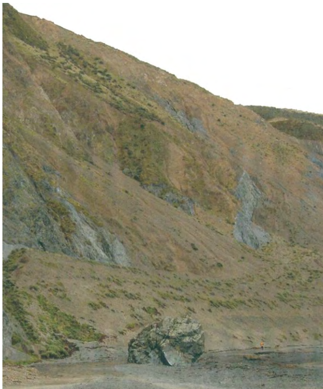
Quarry batters unable to be re-shaped are left to create scree slopes, then spray with native seeds mix.
