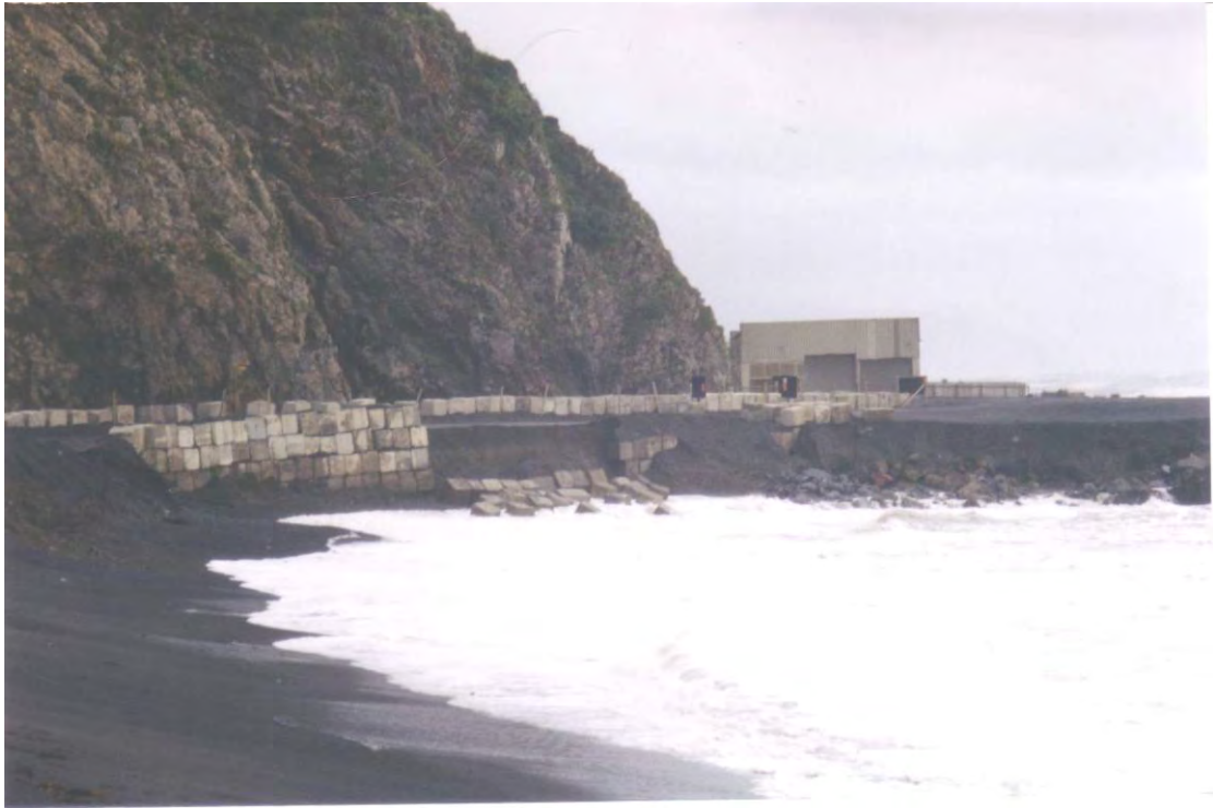
Concrete block seawall under threat as southerly breakers roll in.
