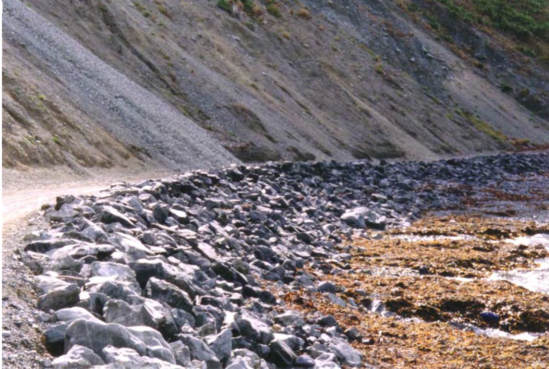
Using surplus riprap (rocks) from the quarry, a sea wall was constructed along the bunded area as a protective shoulder. Western boundary area sea wall is shown.
