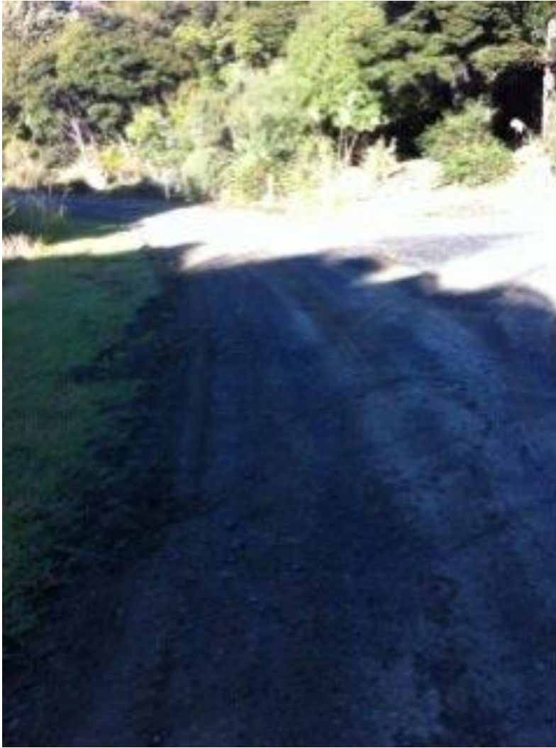
This photo is looking back towards the Wharf ( start of the road ) – extremely bright sun , and to culvert number 6 – the replaced structure. There is a recent access at photo right
