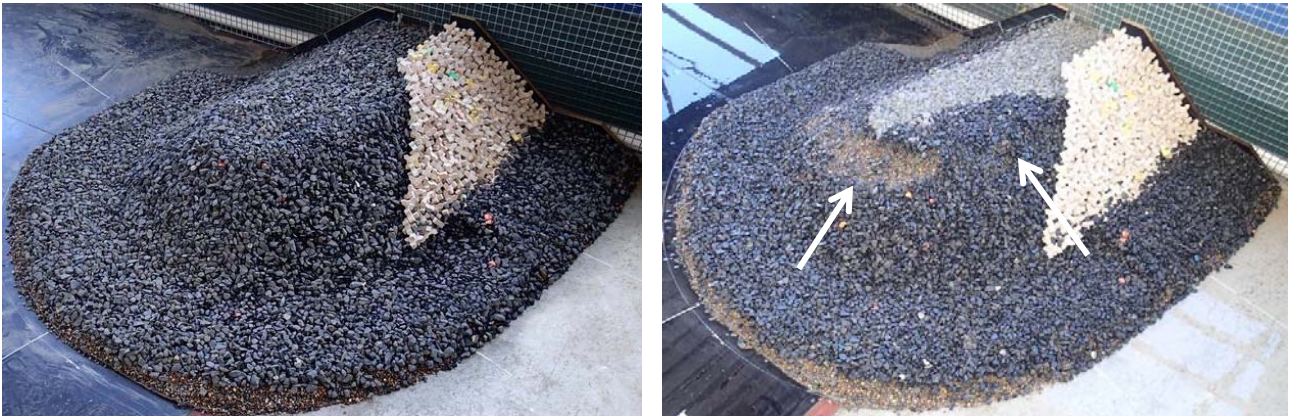
Figure 4. Secondary Armour Stability During Construction: Before (Left) and After (Right) Testing. Arrows indicate filter layer visible at the breakwater head and the end of the trunk.
