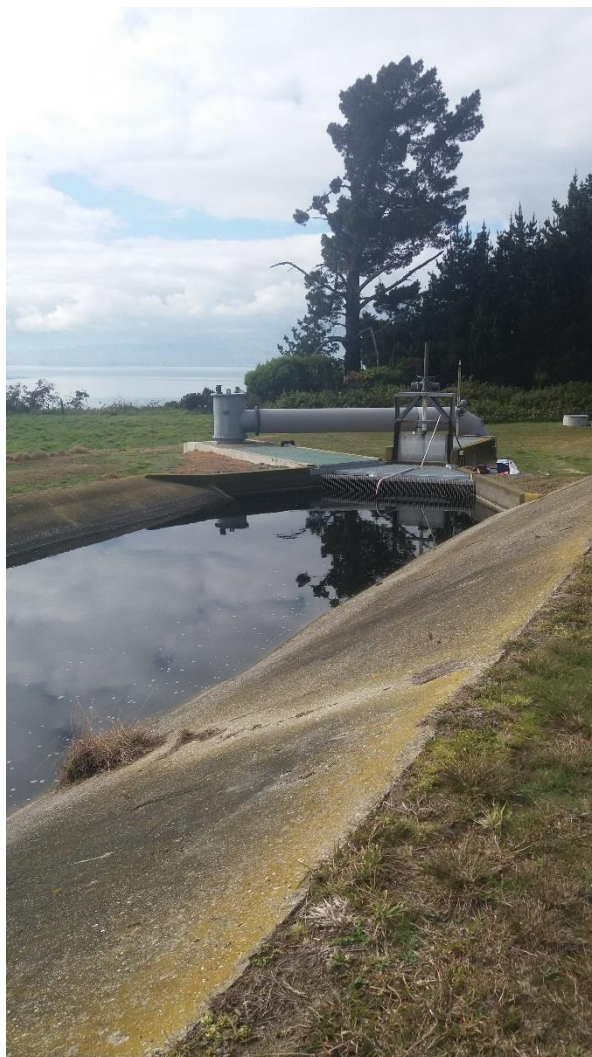
Figure 2. Discharge sampling location, in front of the grating over the discharge pipe.
