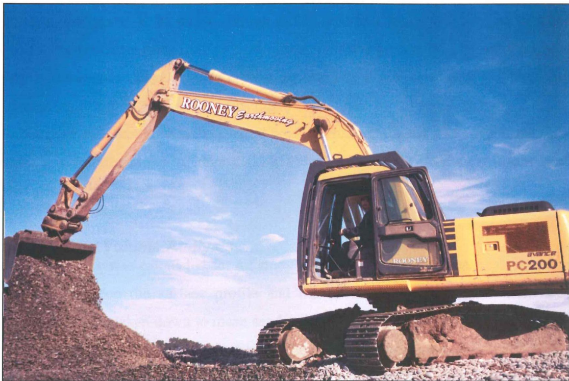
Figure 4.3: Photo of the Digger (Rooney Earthmoving) used to excavate the pits and trenches on the Waihao-Wainono Barrier.
