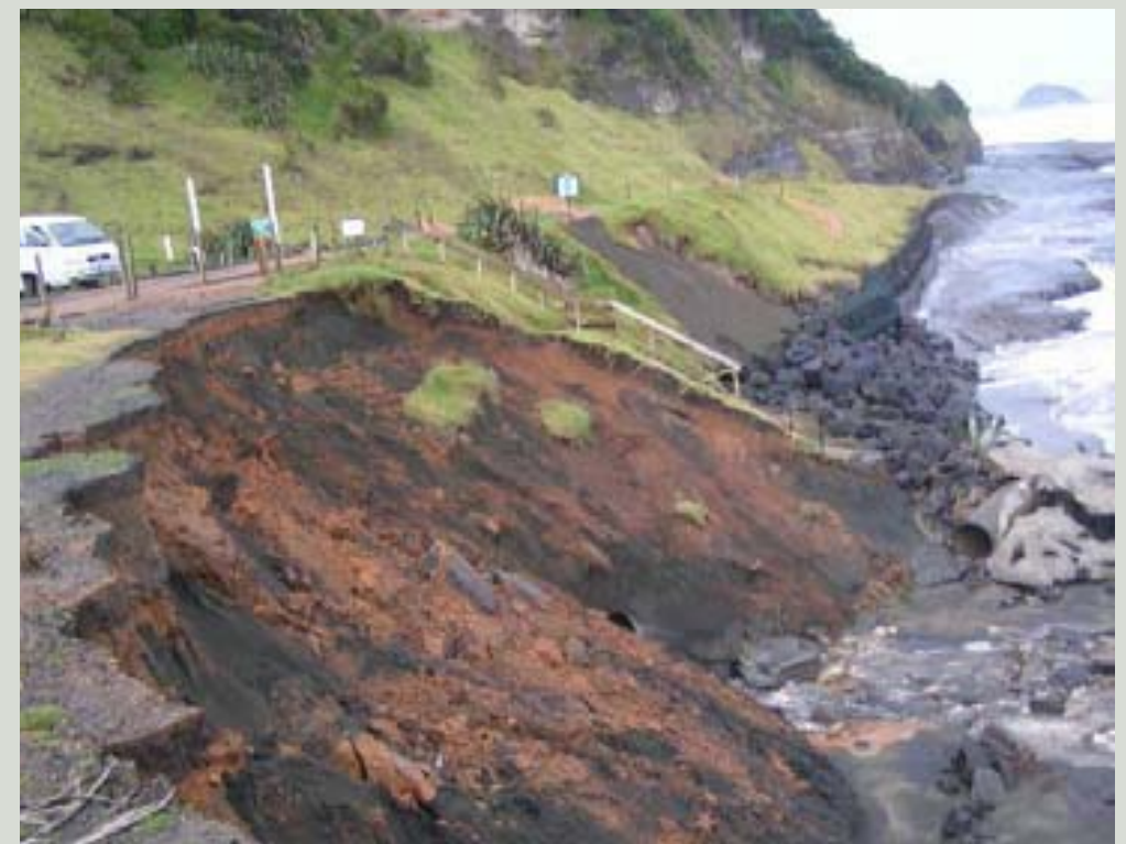
Main car park and arrival area damage
