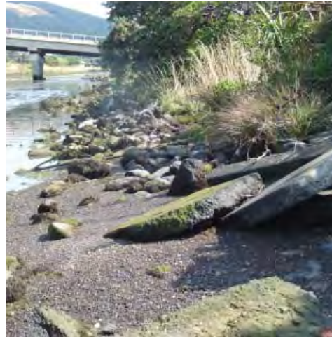
Concrete debris along Porirua Stream
