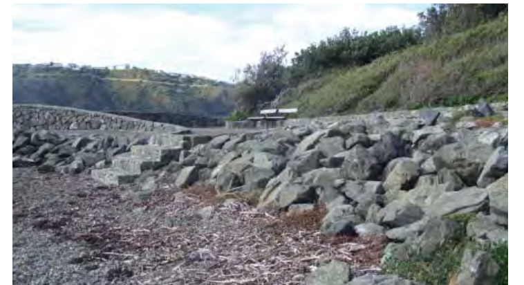
Boulder wall being colonised by planting, with promenade and steps - Wellington Harbour Greta Point
