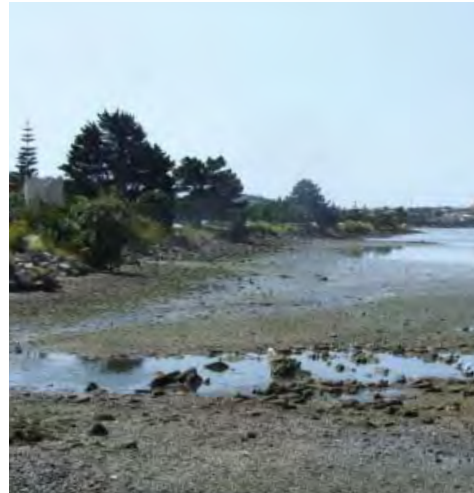
Riprap edge washing out into the harbour floor
