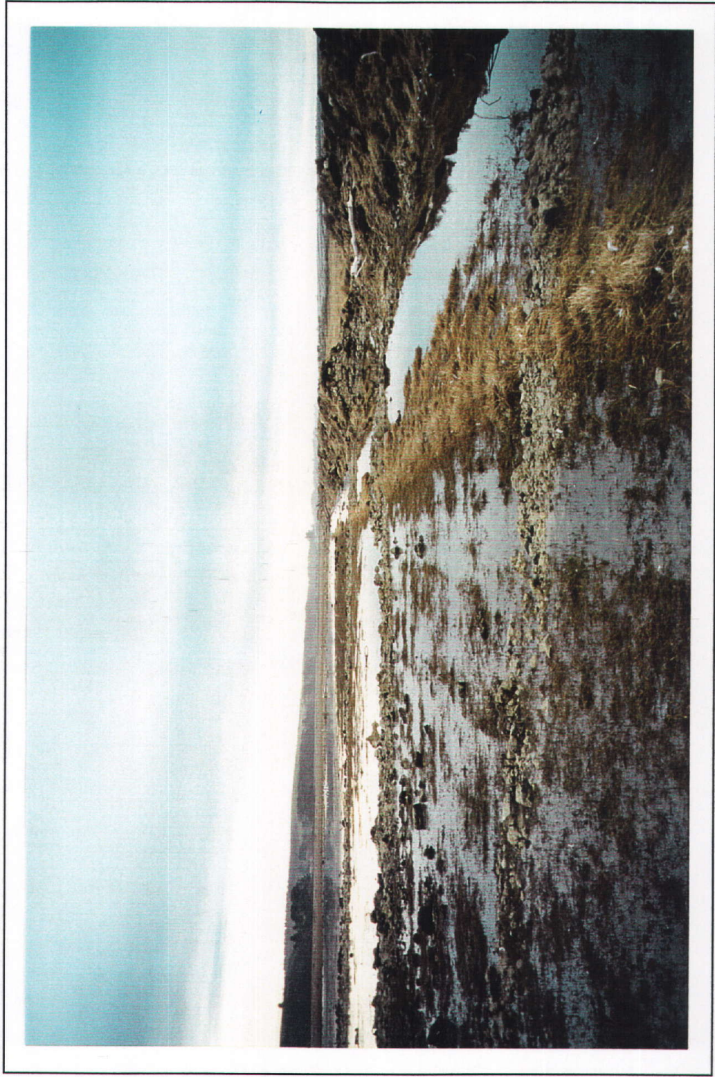
Figure 6.8 Significant damage to unconsolidated stopbanks south of Otaio River.
