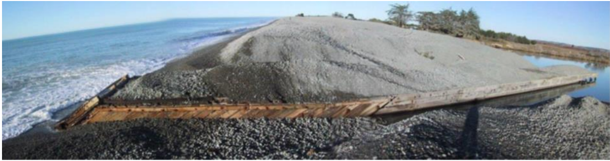
Figure 2-3: Photo of the Waihao Box outlet. The sea is to the left and the Waihao River is to the right of the barrier. From Stapleton (2005).
