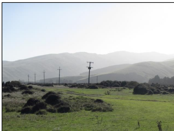
Plate 5: Transformer pole and other power poles next to main vehicle access track.
