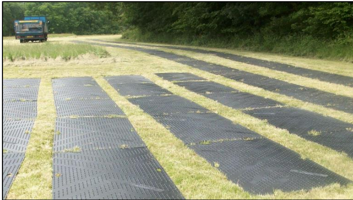
Plate 29: The surface of the proposed landing pad (225 m 2 ) will be covered in temporary materials such as outdoor flooring mats (photo from Ladley 2017). The pad will be no higher than 150 mm off above the ground.
