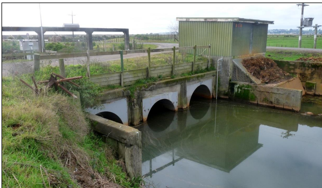
Figure 9: Outlet of Ford Road drain showing pumping station
