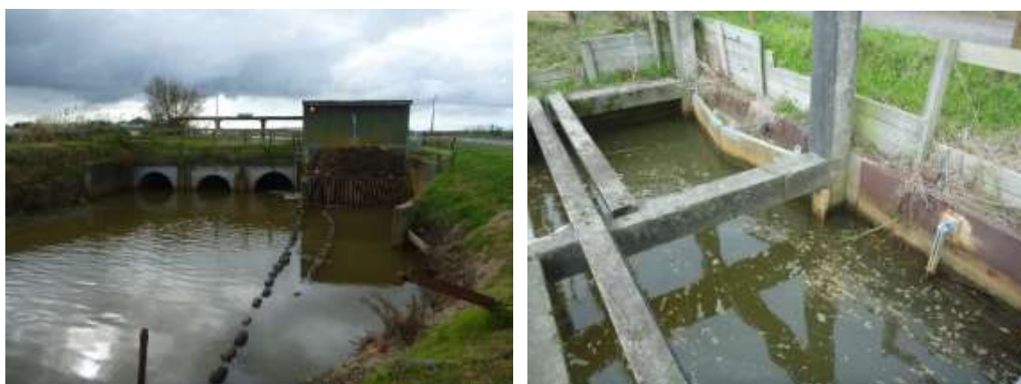
Figure 2 Outlet end of Ford Rd Drain to river showing drain (upstream) side on left and river (downstream) side on right. In the left hand photo the pumpstation and its intake grill can be seen to the right of the culverts. At this time the river level was high and the flapgates were closed
