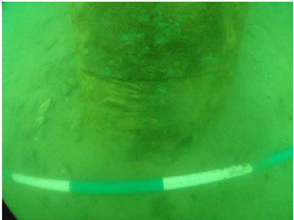
Original wharf pile showing copper sheathing
