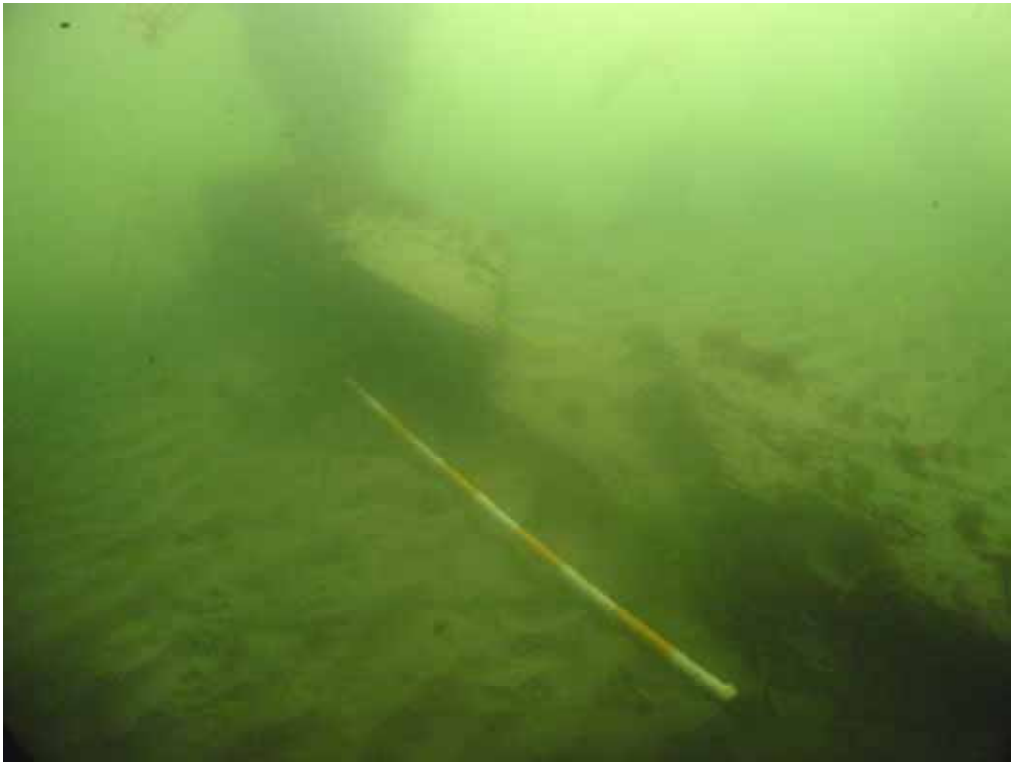
Fallen timber cross beams on the seabed below the wharf
