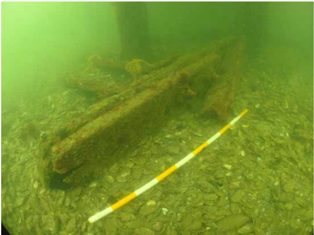
Fallen wharf timbers on seabed at seaward end of wharf, August 2012
