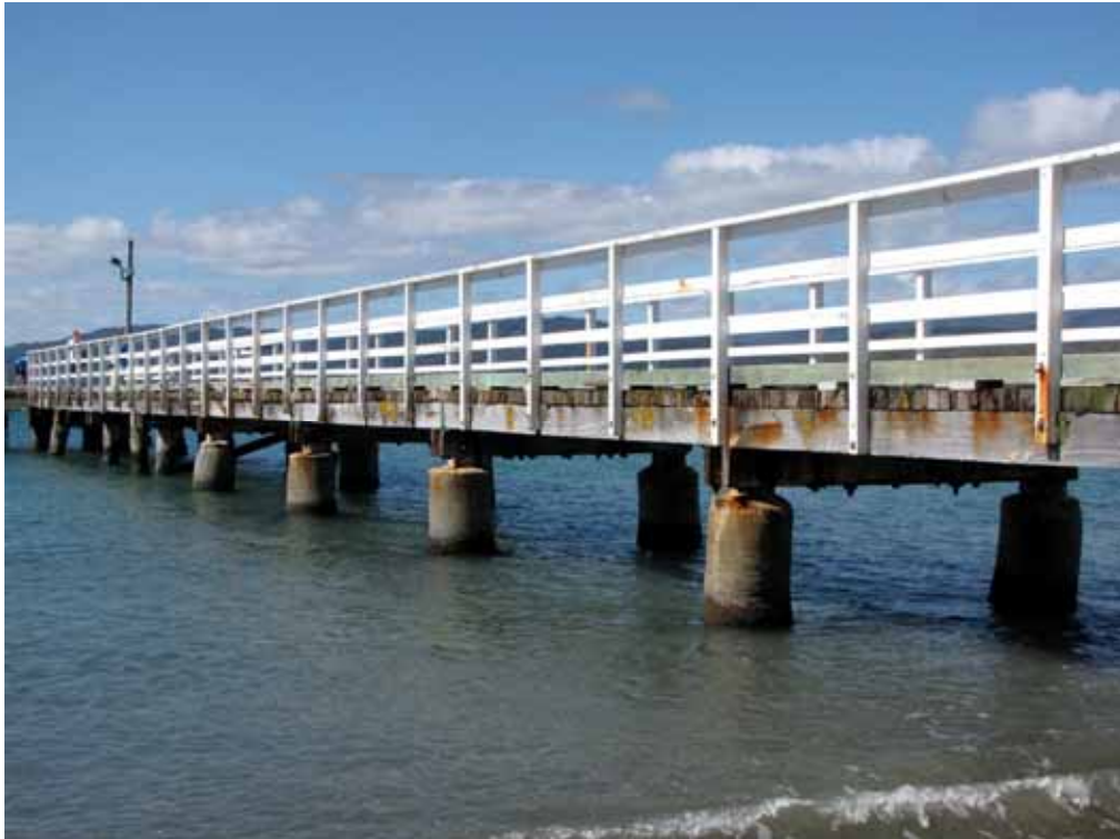
Close up view of the west side of the wharf; strengthened piles in the foreground
