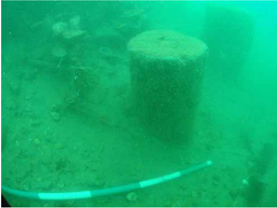
Truncated piles at the outer (northern) end of the Miramar wharf
