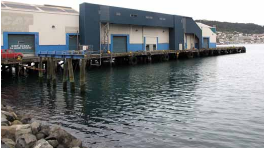
Waterloo Quay Wharf, from the west, 2012. The foreground structure appears to have been part of a ferry loading ramp, probably from the fast ferry operations.
