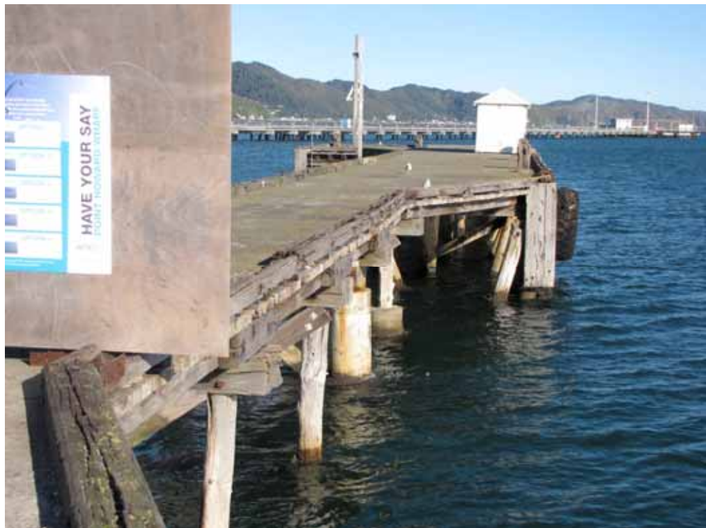
Southern arm of the outer T of the wharf, Seaview Wharf beyond.
