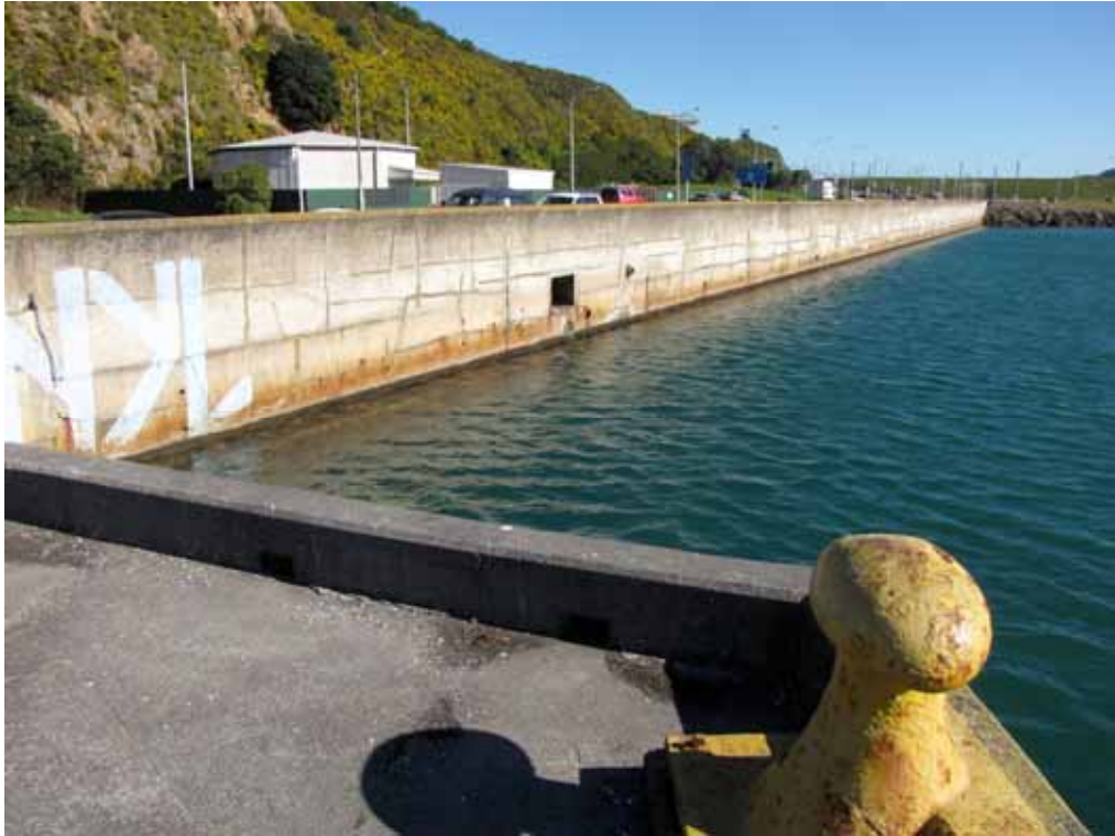
The seawall to the south, known as Aberdeen Quay, Cobham Drive above.
