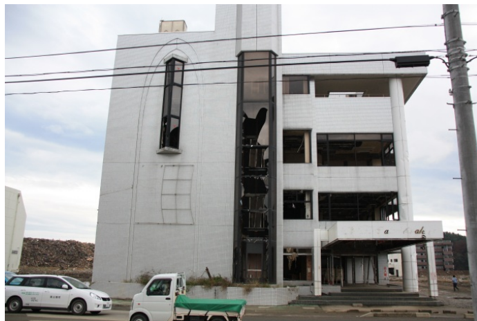
Figure 56 The Takano Kaikan building 160 m inland of the Matsubara apartment block. Little damage aside from glazing was observed here, despite heavy damage and collapse of RC buildings immediately seaward.
