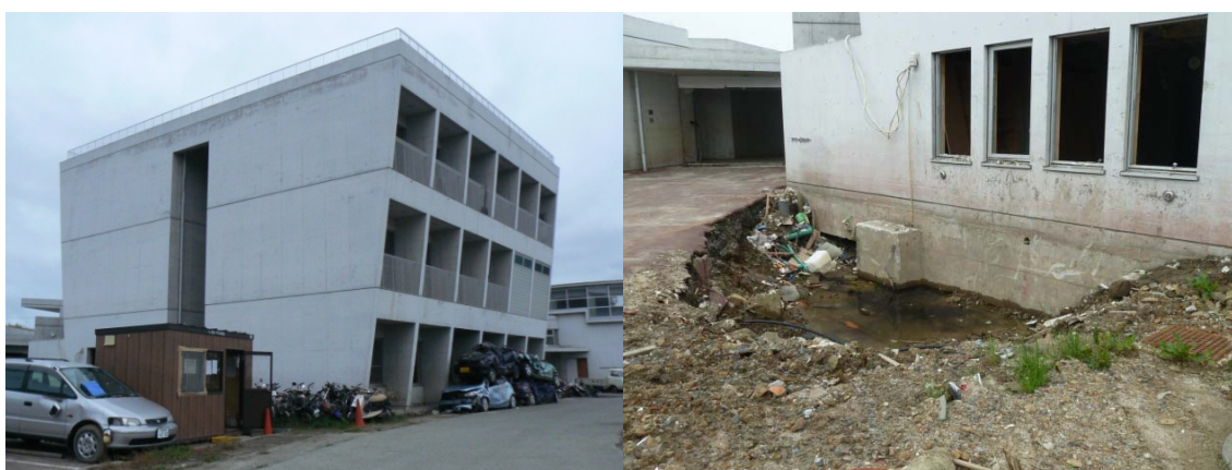
Figure 48 An elderly persons' welfare centre which was inundated to around 8 m height. Scour up to 2 m deep occurred on the near side of the building in this photograph. Extensive damage occurred immediately inland of this building, while 80 survived on the upper floors.
