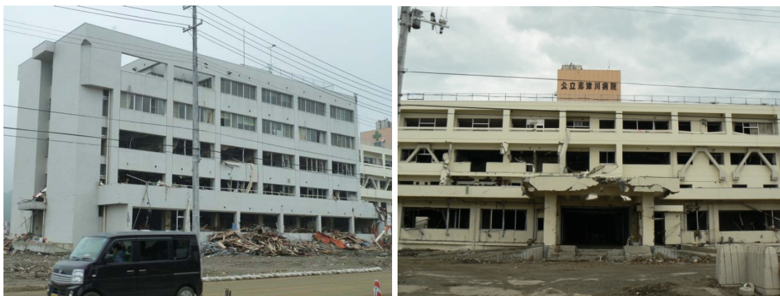
Figure 57 Shizugawa Hospital (west building) – the taller of the 2 hospital buildings at 5-storeys, this section suffered less debris damage than the east building.
