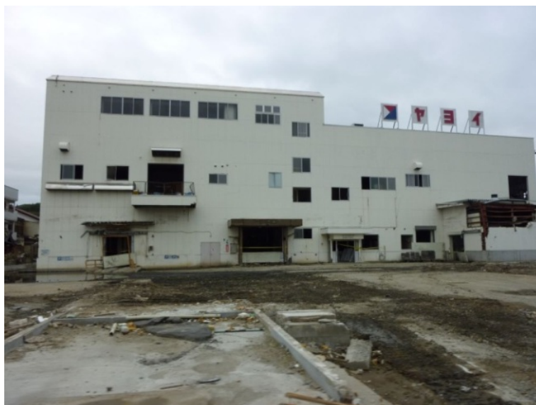
Figure 47 The Yoyoi food factory, where 400 people took refuge. Inundation height was around 8 m here.
