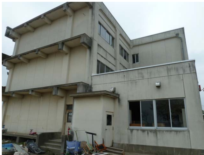
Figure 67 Yuriage Junior High School is constructed on ground which is raised 1.8 m above the surrounding fields. This helped to mitigate damage from the tsunami flow and only contents damage was observed (EEFIT, 2011). 823 people took refuge here.
