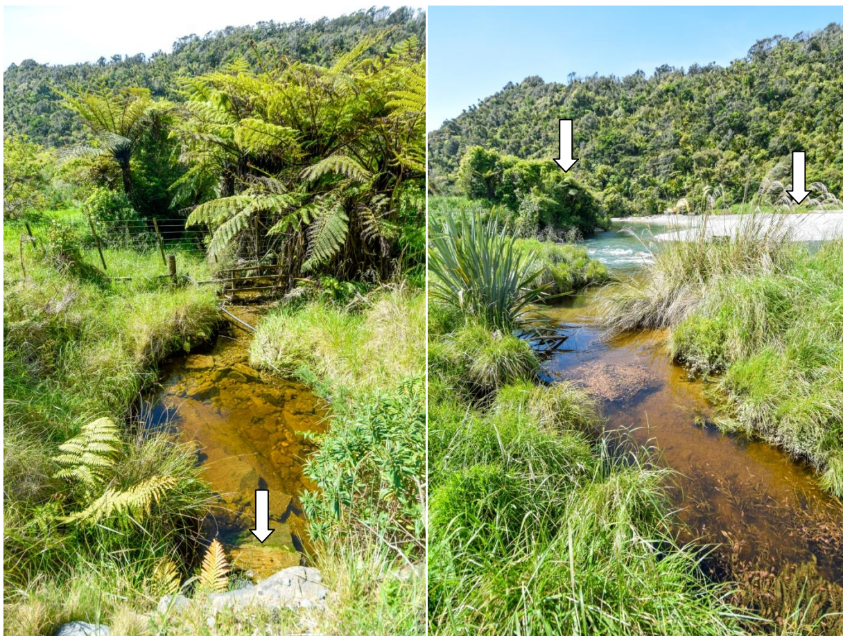
Fig. 3. (a) Pool below the perched culvert (arrowed) at Waikori Road. (b) Stream confluence with the Punakaiki River showing position of bridge abutment armouring (left arrow) and gravel extraction activities (right arrow).
