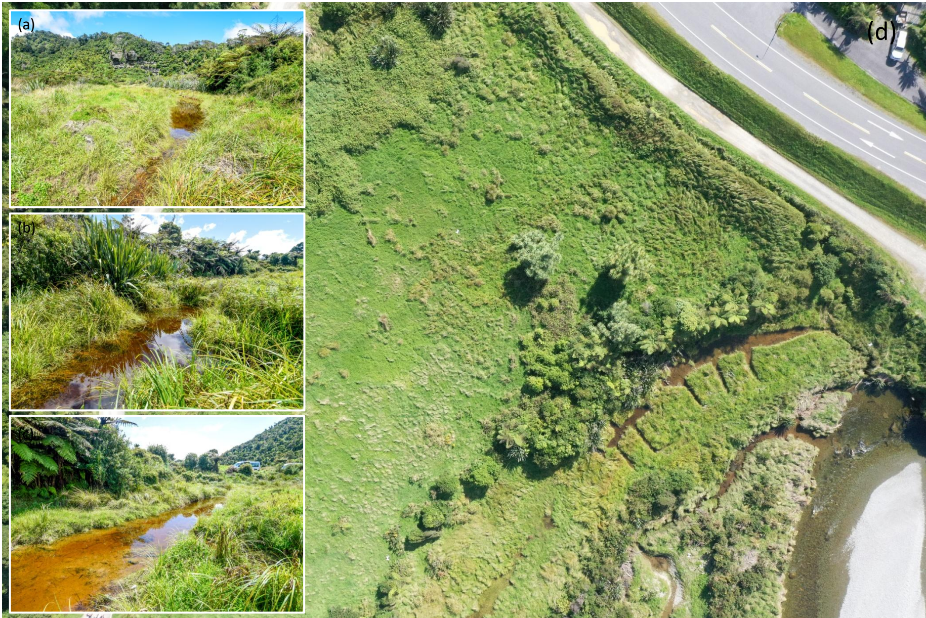
Fig. 5. (a) – (c) three views of engineering works on the stream confluence terrace. (d) aerial view showing location of the works. Note close proximity to picnic area access point to the north.
