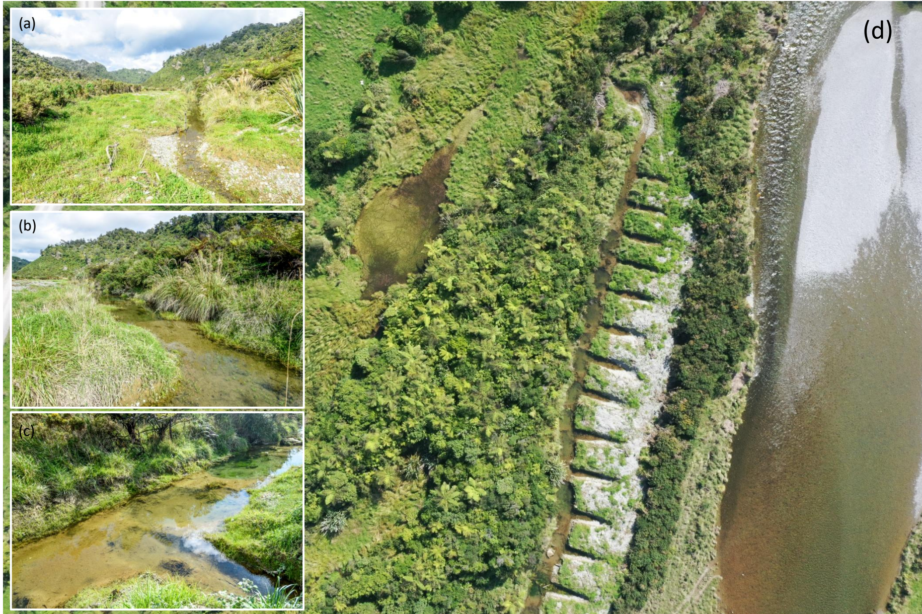
Fig. 4. (a) – (c) three views of the old channel engineering works. (d) aerial view showing alignment of the channel and existing forest remnant on the western bank.
