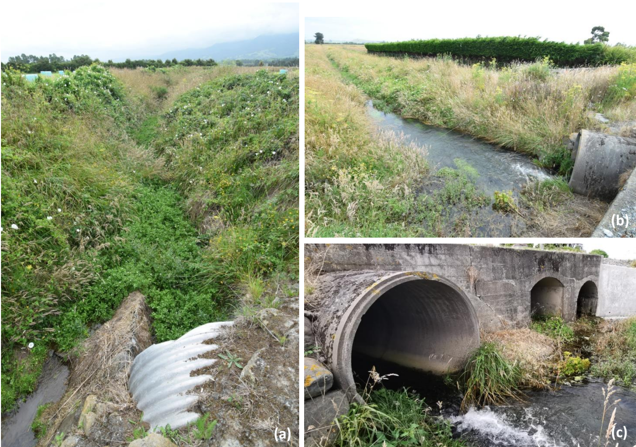
Fig. 7. (a) Luke Creek upstream of Burrells Lane. (b) and (c) two views of the culvert in Luke Creek at Schoolhouse Road.
