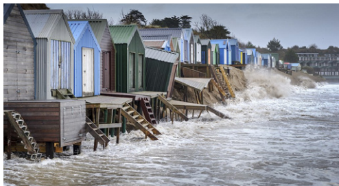
Figure 3. Beach huts were damaged by flood water in Iconic beach, North Wales, UK (Duell, 2014).
