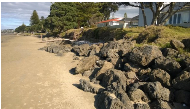
Figure 95. Existing armour failed to prevent erosion in the north of Marine (Tonkin & Taylor Ltd, 2015, p.4).
