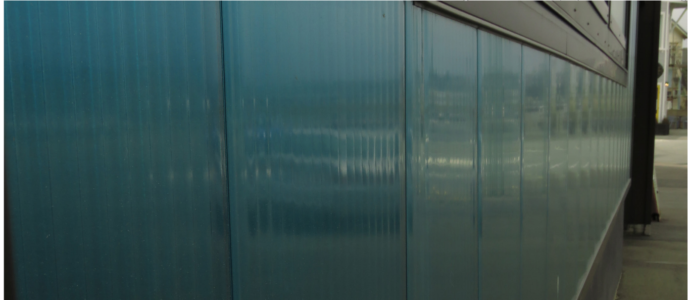
figure 6.9 Rodeca polycarbonate cladding
