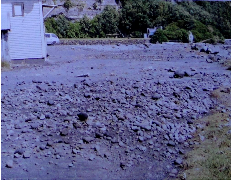
Figure 18 The aftermath of wave overtopping the seawall during a storm event in February 2018. Mr Brian Vincent's photo.
