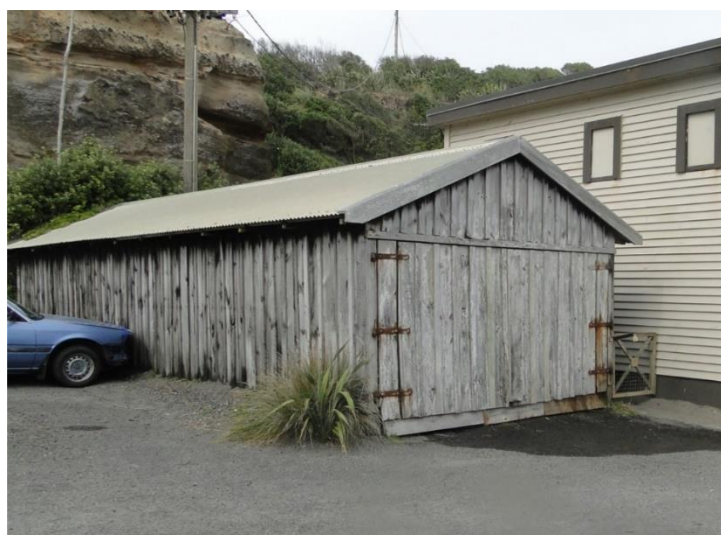
Figure 8 The top photo shows 3 boat sheds undermined by the March 1999 storm (source: Taranaki Daily Mail, 19 April 1999). Note rubble littering the beach – this was originally placed against the bank to provide wave protection. Lower photo shows the last remaining boat shed at 16 March, 2020.
