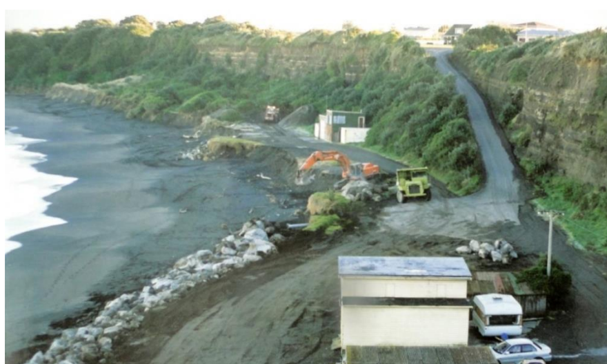
Figure 9 Upper photo: pouring concrete for the boat ramp, May, 1977 (Mr Brian Vincent photo). Central photo: constructing the (present) ramp wall using concrete blocks, c. 1986 (Mr Brian Vincent photo). Lower photo: constructing the current rock revetment in July 1999 (Mr Gerald Bourke photo).
