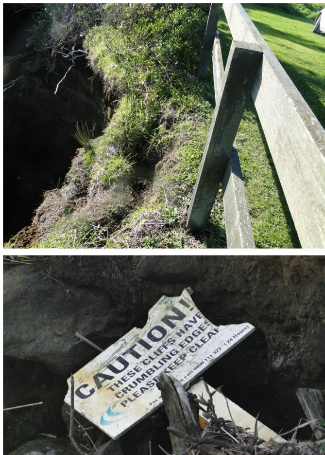
Figure 20 Southeast cliff stormwater gully showing the upper edge, barrier fence and state of the warning sign in May 2020.
