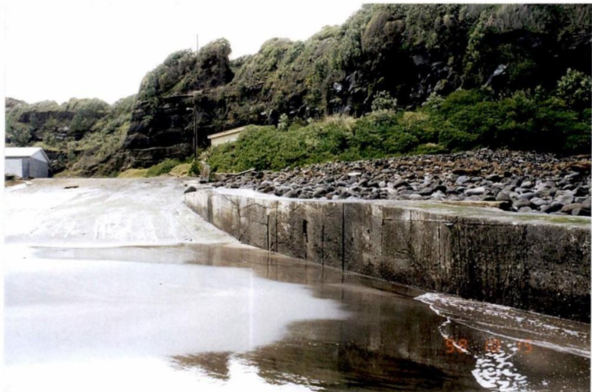
Figure 5: Concrete boat ramp and groyne, which has trapped cobbles and boulders on the S side (Photo: 15 October 1998).
