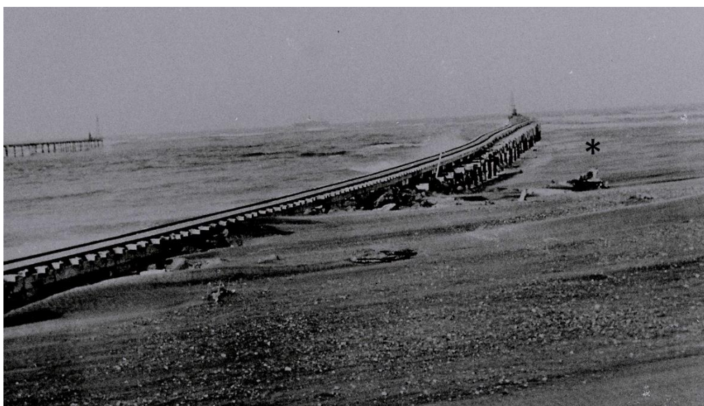
Figure 1 Partially completed moles in the early 1920s raised to high tide level in the foreground and half tide in distance. Sand is washing into the river from the intertidal beach (located by the asterisk) and evidenced by the breaking waves on the river side of the North Mole – this being an indication of lesser depth. At this time the entire South Mole had been only raised to half tide level.
