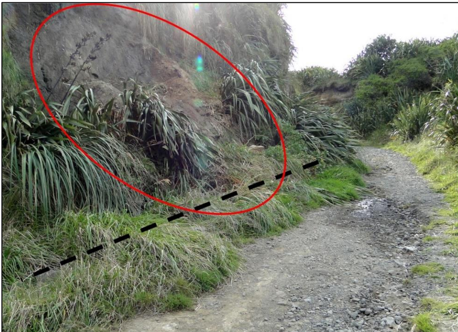
Figure 4.1 Waihi Beach access track showing slumpage (circled) and blocked drainage channel (dashed line) with resulting rills (focused erosion) developing on the track
