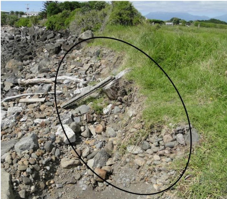
Figure 2.8 Exposed upper bank at southern end of seawall (260 to 275 m).
