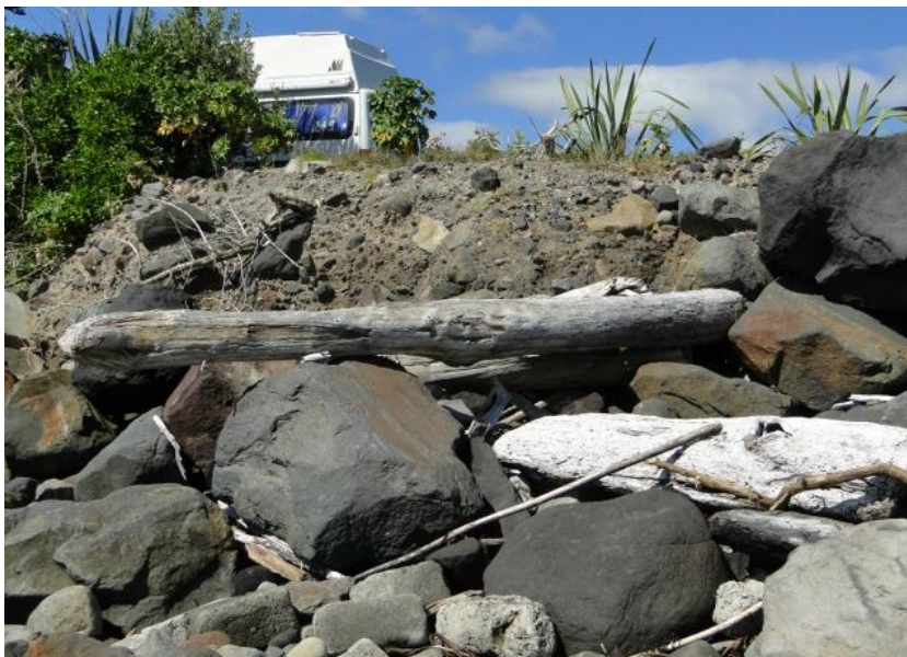
Figure 2.6 Unconsolidated and erodible material at the northern end of recent rock placement at 140 to 150 m chainage.
