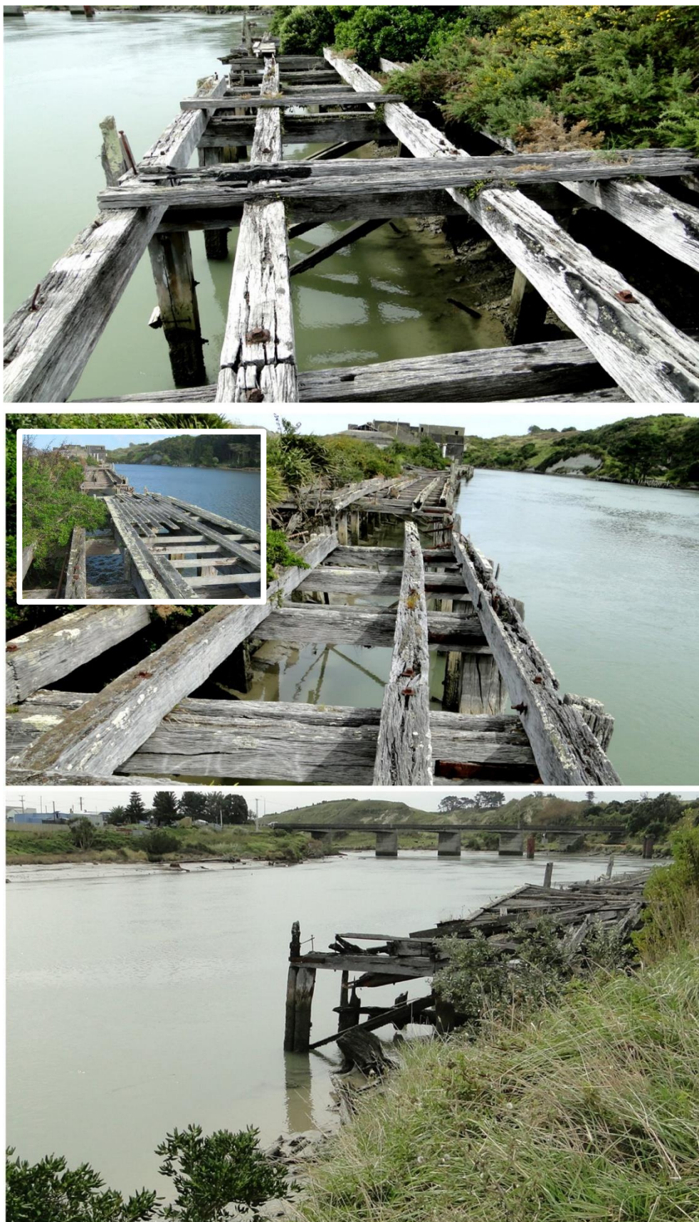
Figure 5.3 Upper photo: upstream section of dilapidated wharf 250 to 200 m. Middle photo: superstructure 290 to 350m, inset for comparison is TRCs 2013 photo. Lower photo: collapsing structure at 360 m with no wharf having been constructed along the next 50 meters.
