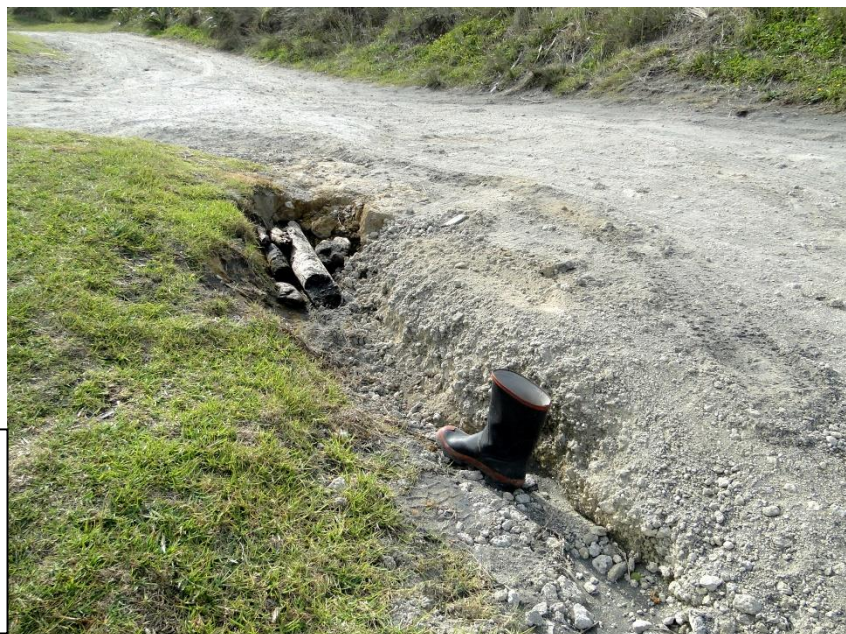
Figure 6.5 Stormwater drainage issues above the structure.
