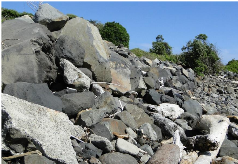
Figure 2.5 Overly steep recent rock placement at 150 to 180 m chainage
