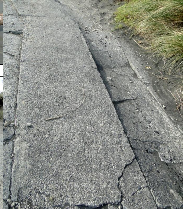
Figure 6.3 Degraded condition of the beach access ramp.
