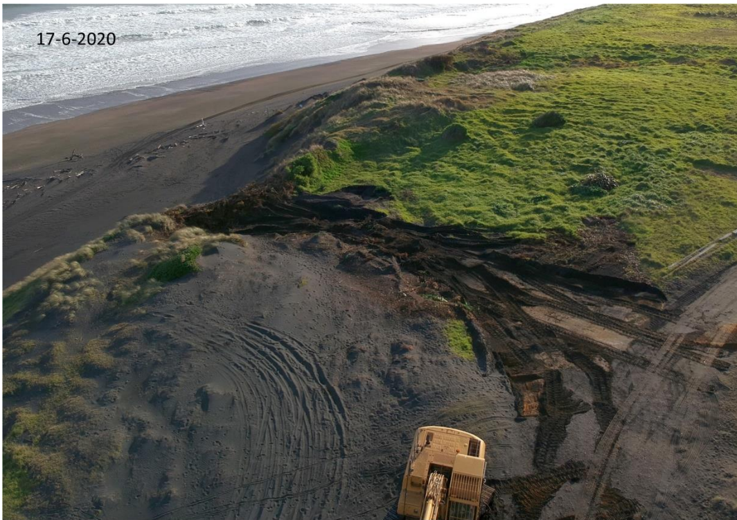
Figure 5 Surface disruption by digger during green waste placement.
