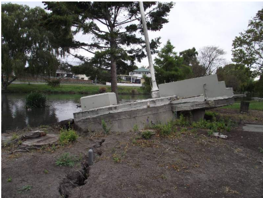
Figure 2.4 Buoyancy of a pump-station floated up to 500 mm out of the ground by liquefaction adjacent to the Avon River near the eastern end of Morris Street, approx. 10 km from the epicentre after the magnitude 6.3 Christchurch earthquake of 22 February 2011. (Photo: D. Beetham, GNS Science).
