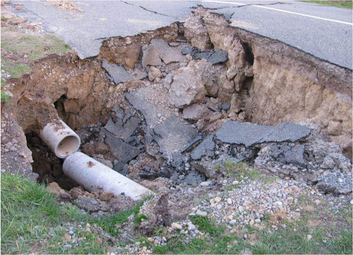
Figure 2.8 Damage to underground infrastructure from liquefaction, in this case lateral spreading has pulled a pipe joint apart in Cashmere after the magnitude 7.1 Darfield earthquake of 10 September 2010.
