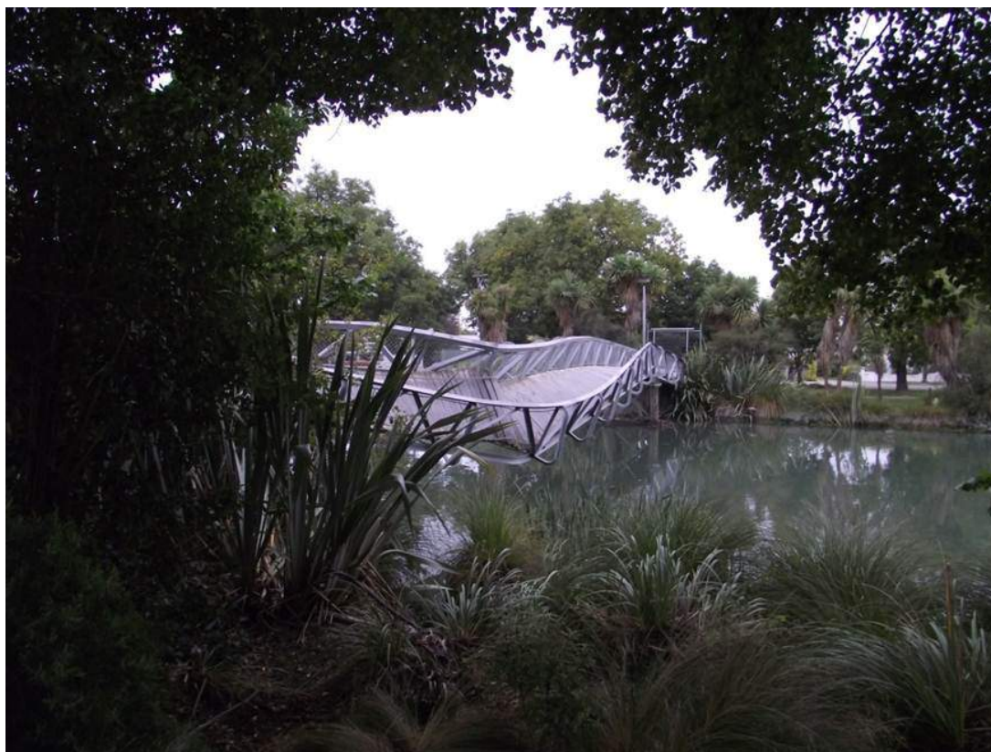
Figure 2.6 Compression-induced buckling of a bridge over the Avon River near Medway Street due to lateral spreading displacement of the abutments approx. 10 km from the epicentre after the magnitude 6.3 Christchurch earthquake of 22 February 2011. (Photo: D. Beetham, GNS Science)
