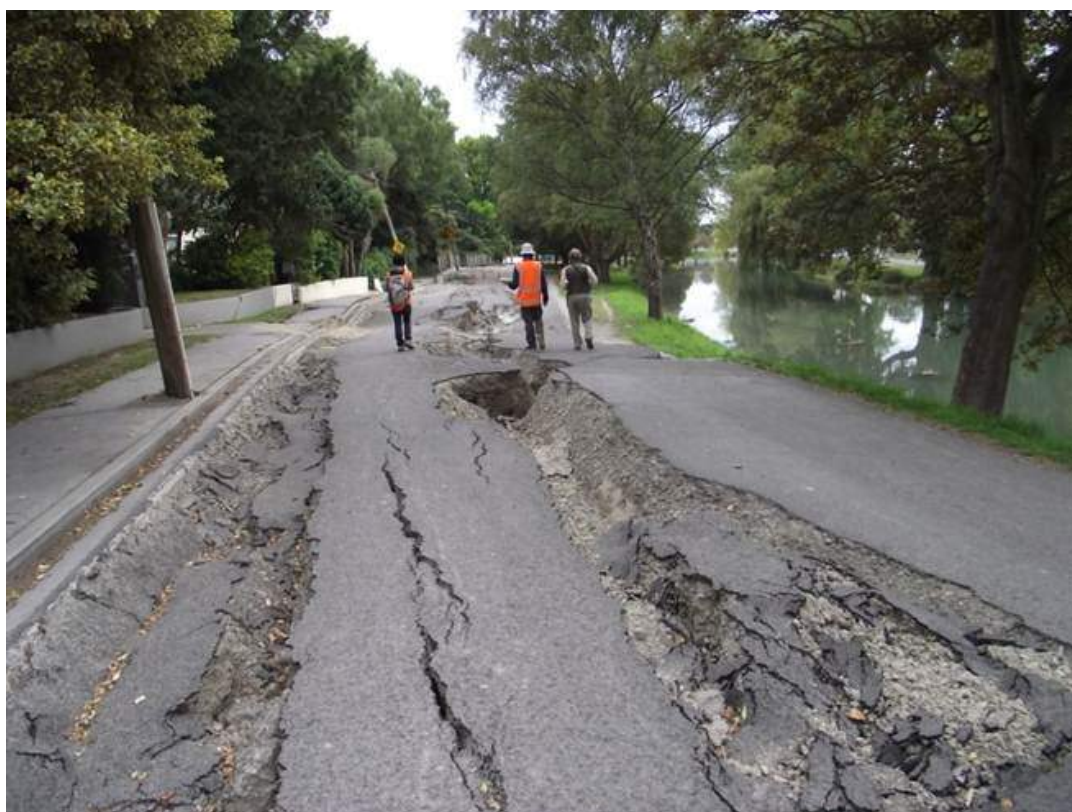
Figure 2.5 Lateral spreading fissures run parallel to the Avon River in Avonside Drive, Christchurch, approx. 10 km from the epicentre after the magnitude 6.3 Christchurch earthquake of 22 February 2011. (Photo: D. Beetham, GNS Science)
