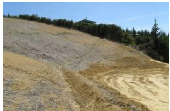
Figure 8-6 Contour drain intercepting slope runoff. Note straw mulch to reduce raindrop impact
