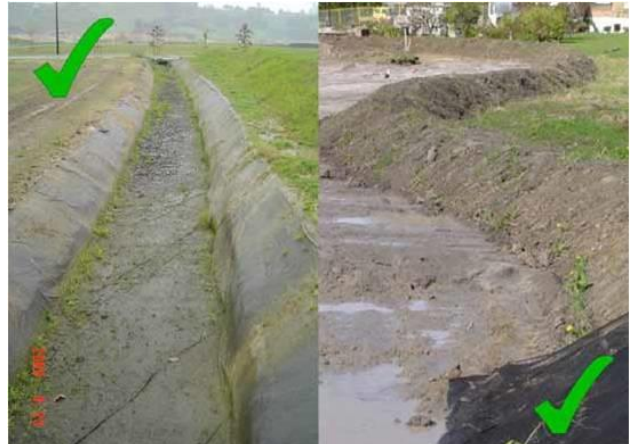
Figure 8-8 Diversions for intercepting clean water (left) and dirty runoff (Photos courtesy of BOPRC and Ridley Dunphy Environmental Limited)
