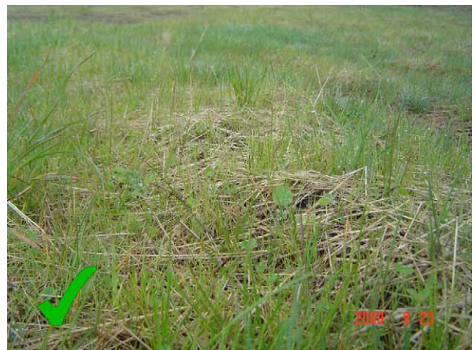
Figure 8-31 Well applied mulch and vegetative cover – photo courtesy of BOPRC and Ridley Dunphy Environmental Ltd
