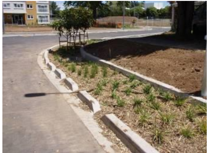
Figure 4-1 Rain garden construction: sediment entry is compromising future performance due to clogging
