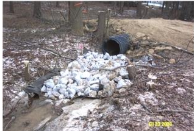
Figure 11-6 Temporary culvert crossing with the rock protection at the outfall to reduce stream erosion
