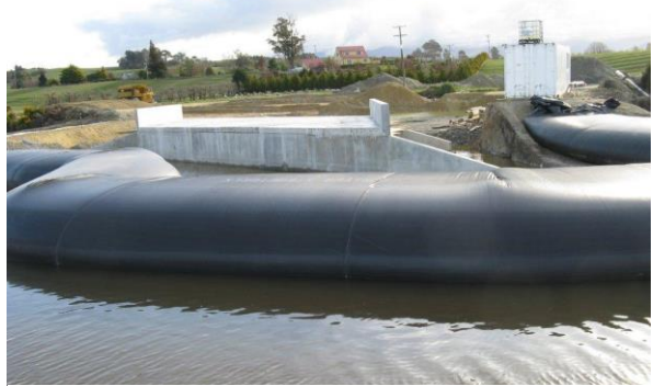
Figure 11-10 Aquadam used on the Ruby Bay bypass to isolate an estuary work site
