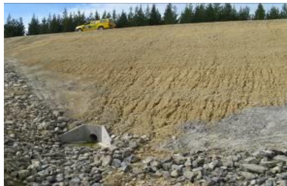
Figure 3-7 Rill Erosion on a Highway Embankment
