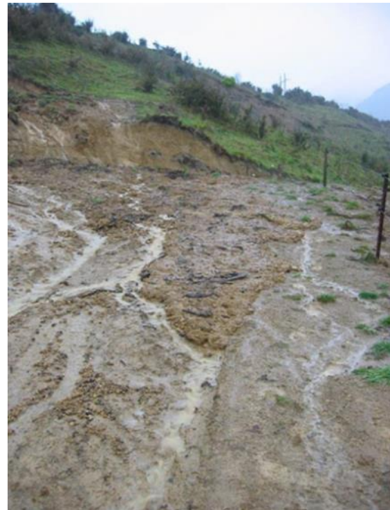
Figure 3-11 Mass Slumping in McConnon Creek Catchment
