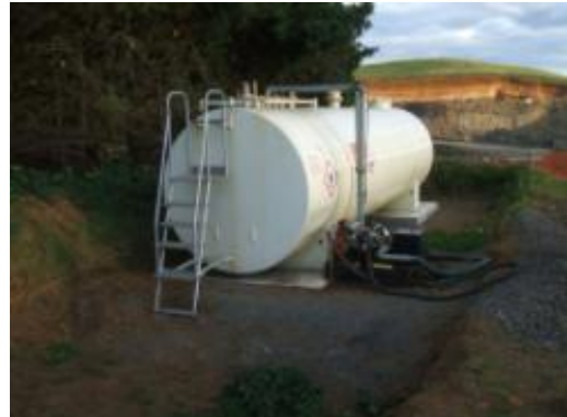
Figure 10-1 Site fuel tank with bunding to contain fuel in the event of a spill
