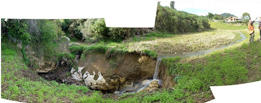
Figure 4-3 Sinkhole in Pohara, Golden Bay draining a waterway from a residential subdivision (Photo: G. Stevens)
