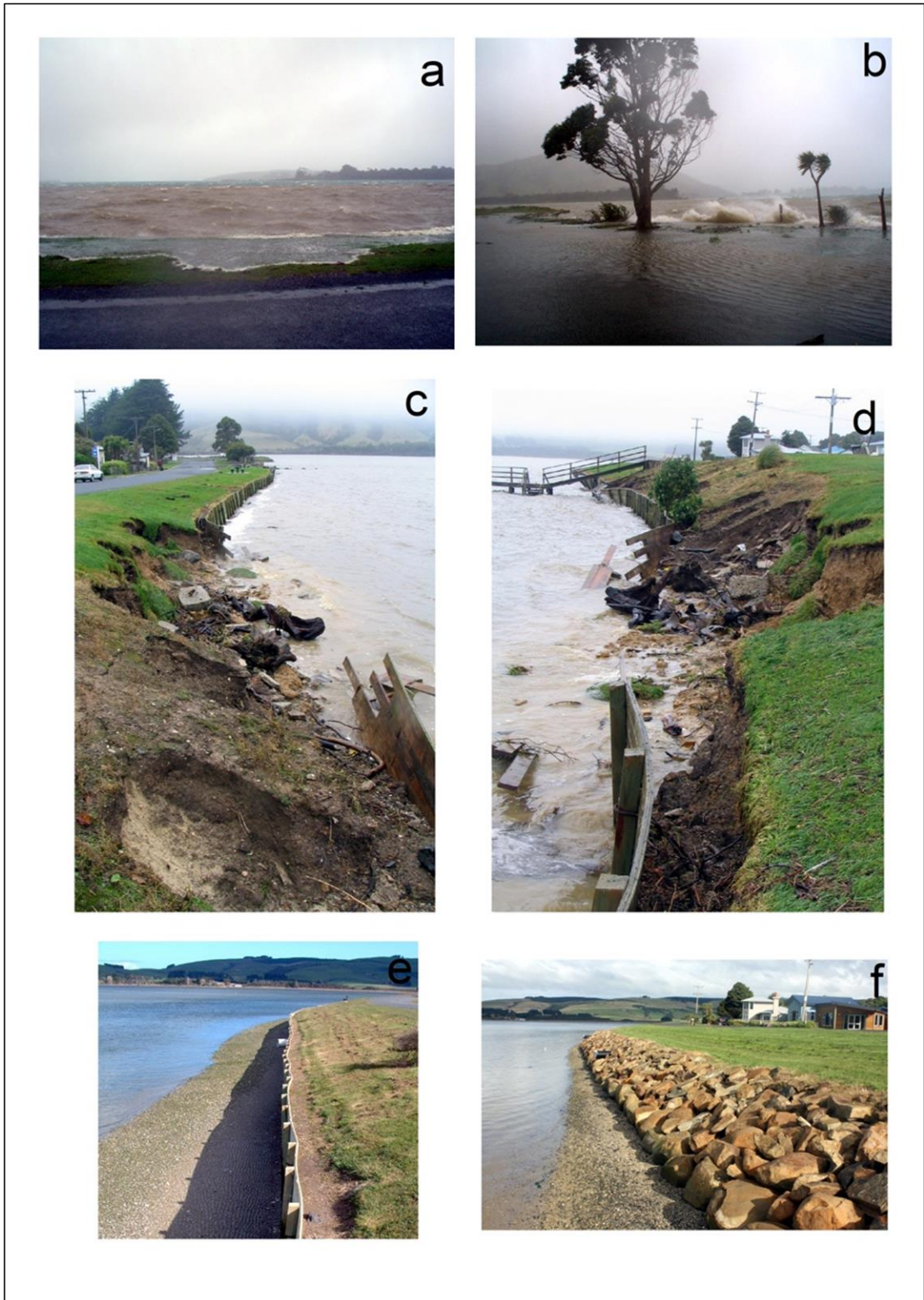
Figure 3.22: Pounaweia foreshore; (a) and (b) wind waves and wave overtopping on April 26 th at high tide; (c) seawall collapse and erosion (looking north); (d) seawall collapse and erosion (looking south); (e) wooden seawall present before 2006 event; (f) rock seawall completed in May 2010. Photos taken by Mike Hilton.
