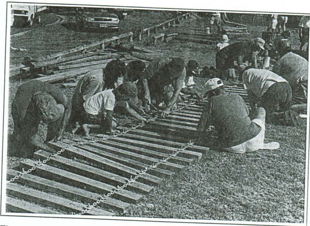
Figure 2a Beach Care group members assembling a board and chain pedestrian walkway.
