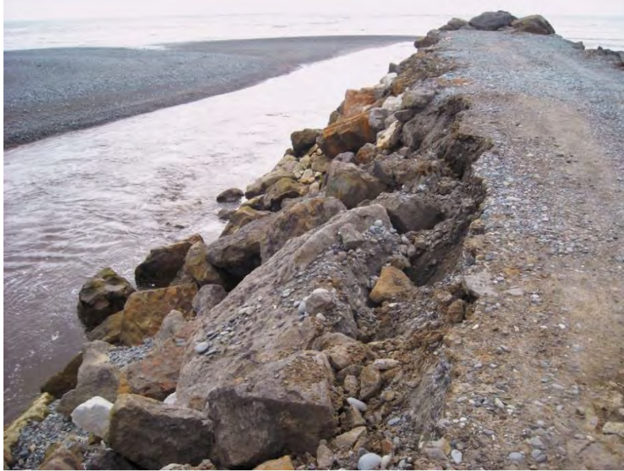
Figure 6.4. Slumping of the southern side of the engineering breakwater at the outlet of the New River Lagoon (27/10/2011)
