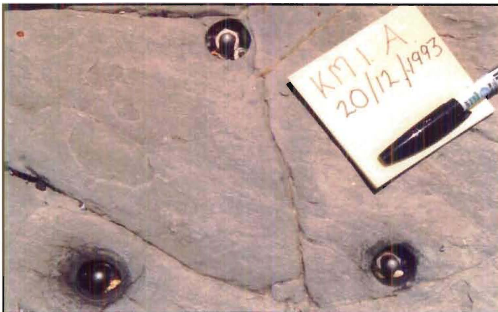
Figure 5.2 A micro-erosion meter bolt site at Kaikoura. Masonry expansion bolts forming the triangle are 150mm apart.
