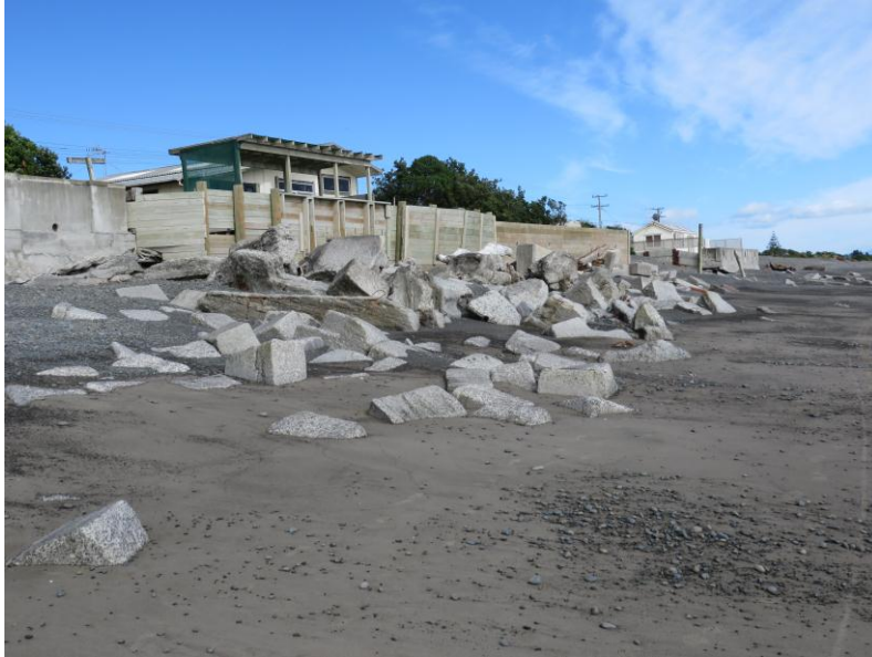
Figure 8: Storm-wave impacts and property damage in the south Haumoana Cell. [Photos from Daykin (2010).]
