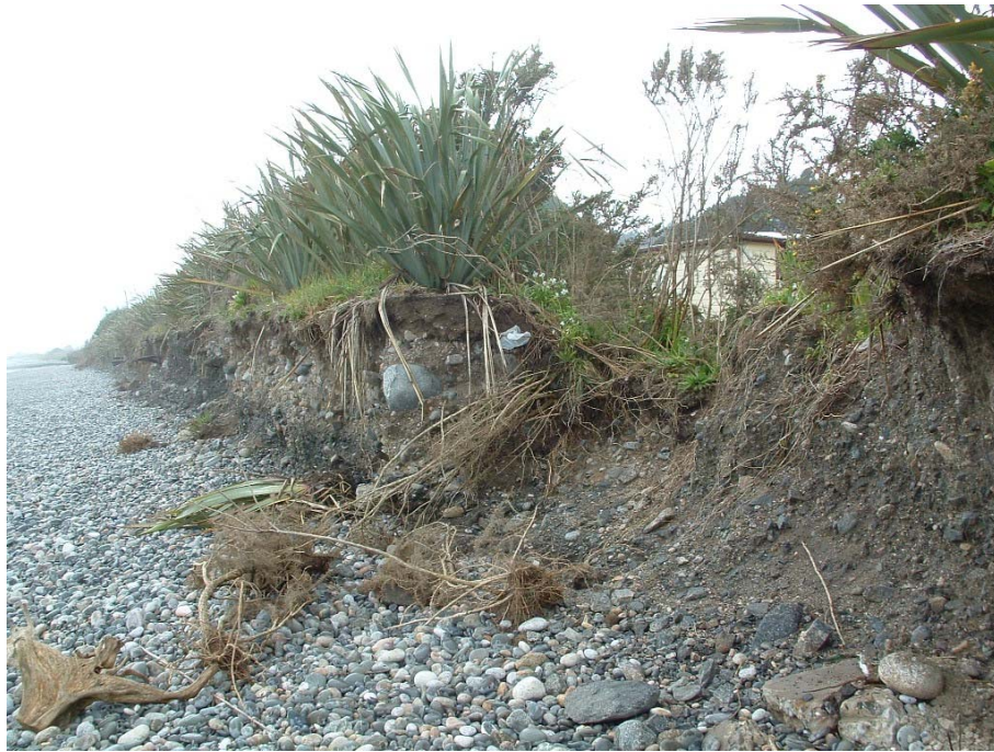
Figure 7: Breach in the stopbank at the southern end of Granity School.
