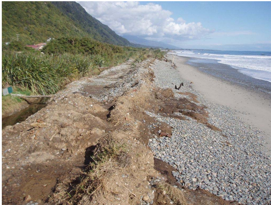
Figure 5: Breached section of stopbank looking south towards Chair Rock.
