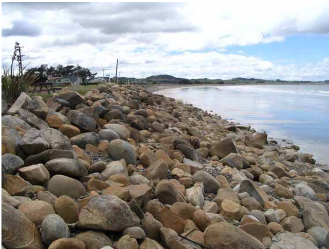
Fig 15a Rock protection awaiting repair - 17 December 2008
