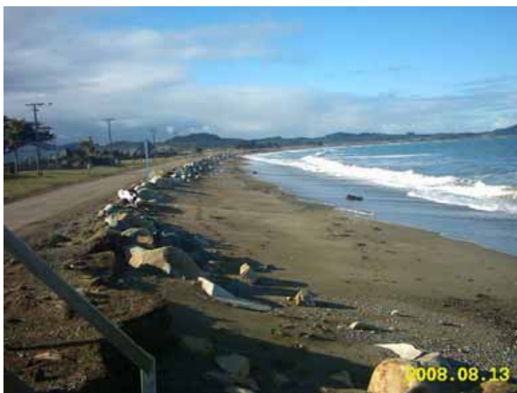
Figure 14a Damaged rock protection, Colac Bay - Photo: Bruce Halligan
