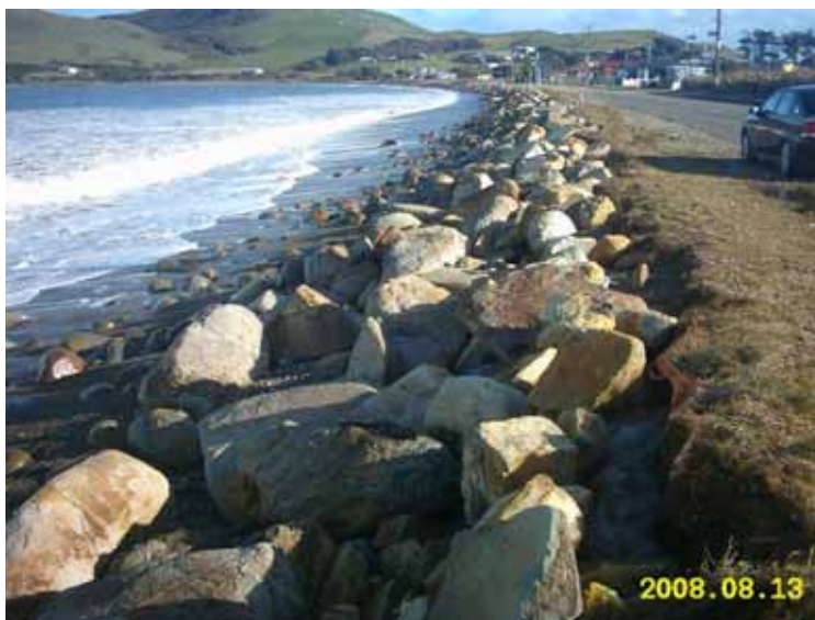
Figure 14 Damaged rock protection, Colac Bay - Photo: Bruce Halligan
