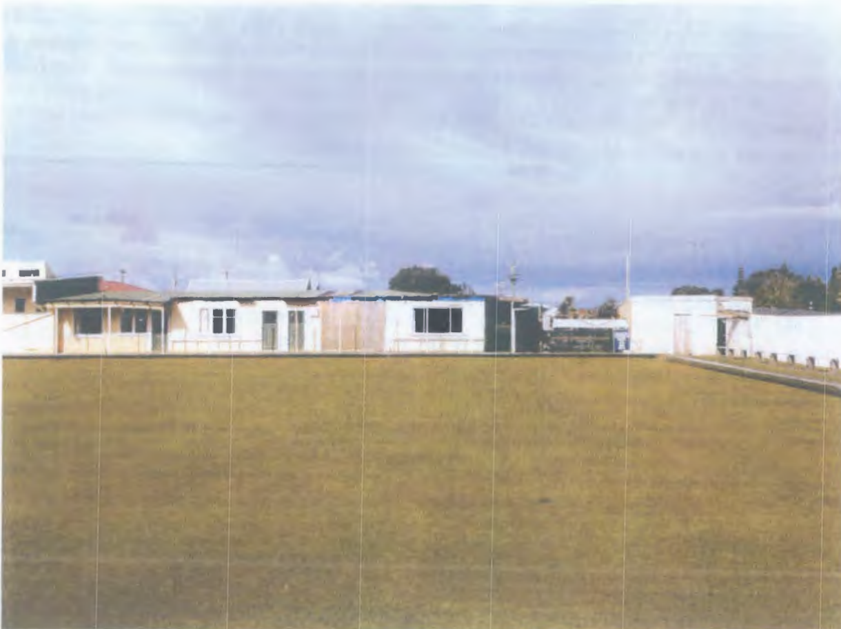
Figure 1.1: View SW across Men's Club green to continuous frontage of club buildings on SE side of green. Women's club house is partially boarded up and temporary tarpaulins utilised to prevent further deterioration from roof damage.
