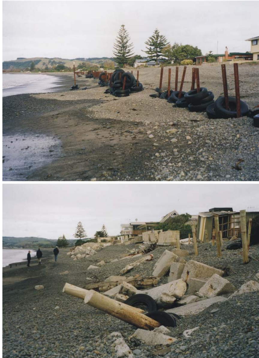
Figure 7-2 The erosion at Te Awanga (upper) and Haumoana (lower), photographed in 2003, with attempts to protect the homes using a variety of shore-protection structures, most of which have failed.
