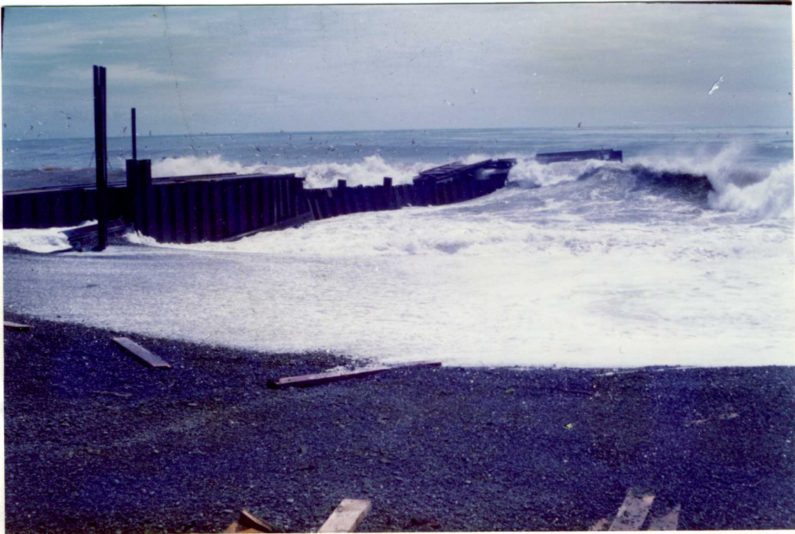
Plate 1 : Wave damage to sheet piling tunnel at the Hastings City sewer outfall, December-January 1979-80.
