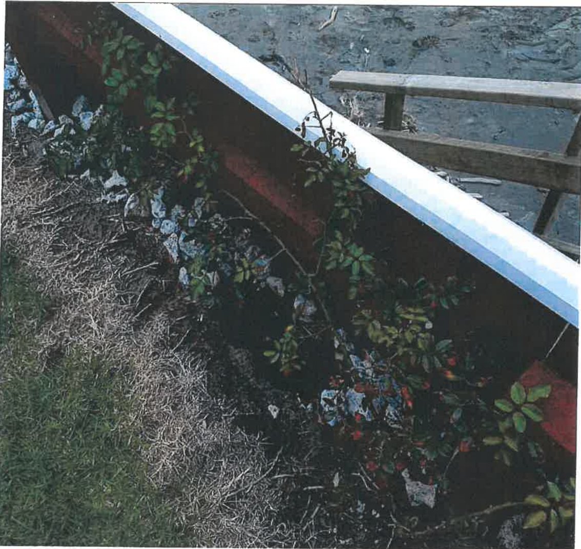
Figure 2: Photo showing voids in behind timber wall at 7 Raebern Lane. The timber wall appears to not have granular drainage backfill or tie-backs.
