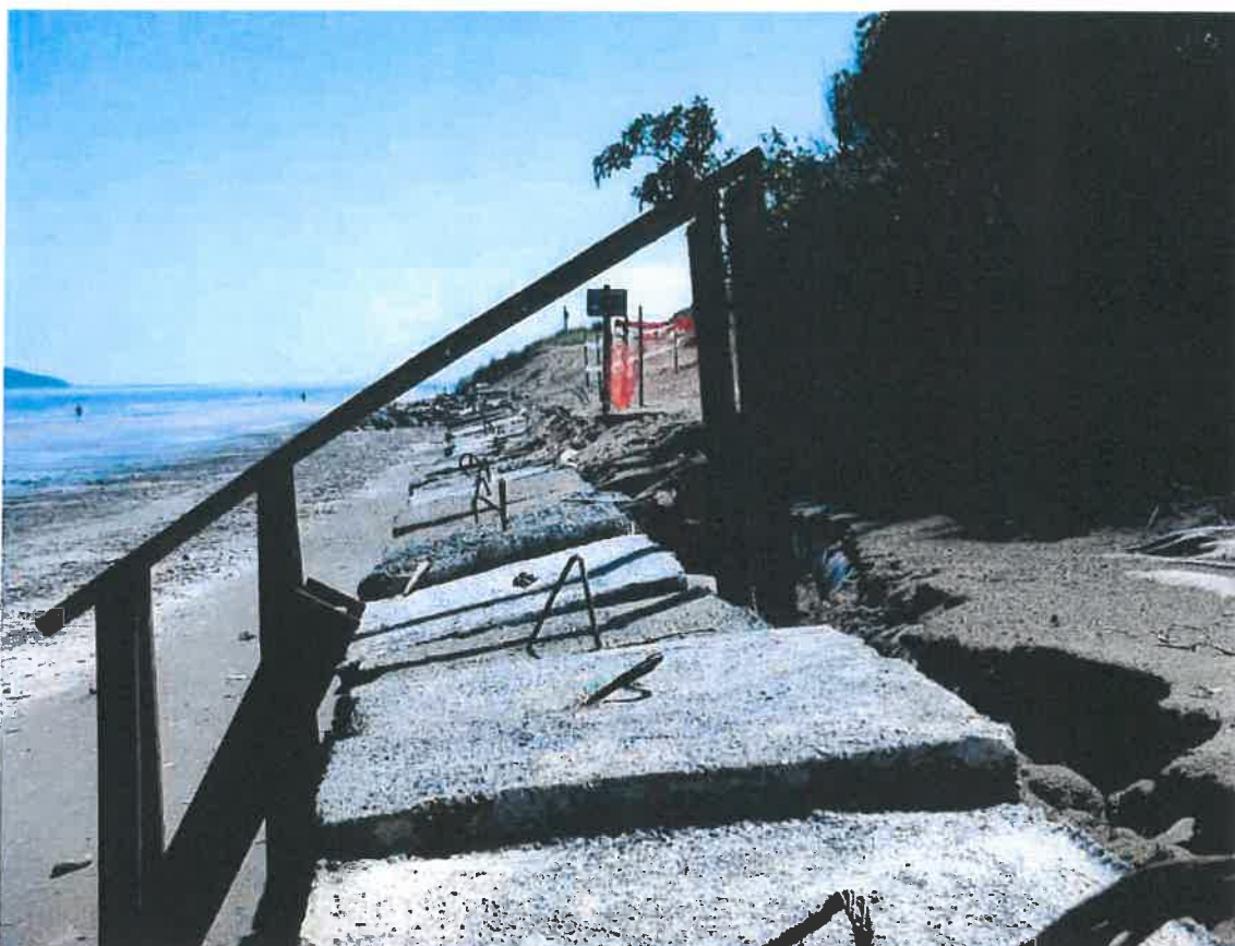
Figure 1: Photo of block wall taken on 20-03-2017 showing seaward rotation of blocks and gap behind blocks exposing bank
