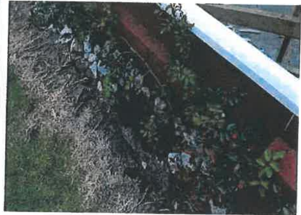
Figure 3 Typical void behind timber wall
