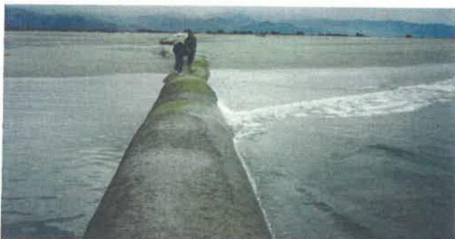
At Port Motueka, sand deflection groyne tubes were used to stop sand build-up in the channel.
