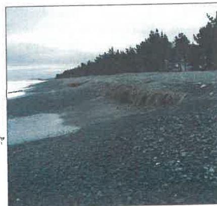
An exposed scarp and extensive scouring of the beach after the October 1993 storm.
