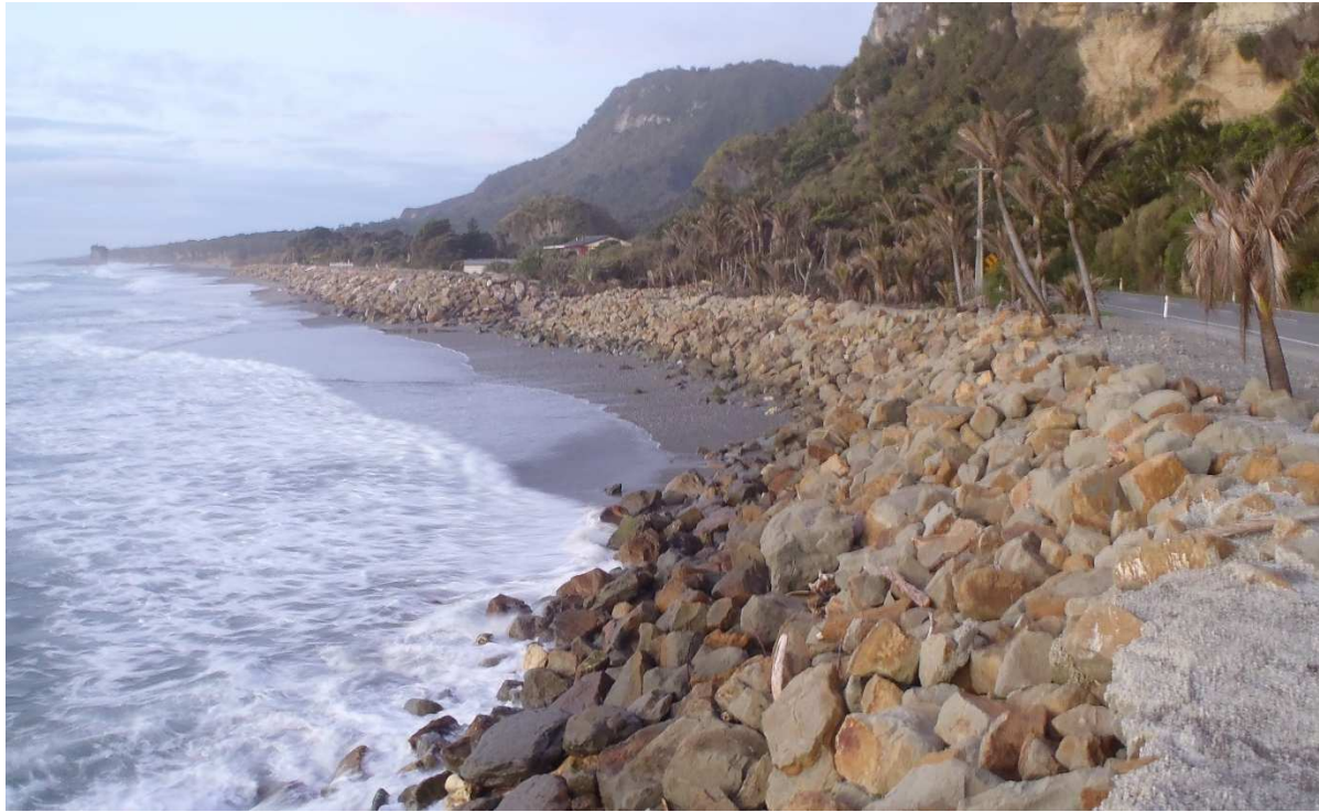
Figure A-1: Larger-scale rock revetment for coastal defence at Punakaiki. Defence constructed to protect both SH6 (visible centre right) and township. Photograph looking north towards Punakaiki township. [22 September 2015].
