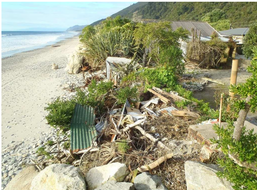
Figure 3-16: Ad-hoc defensive filling of 20 m wide gap in existing revetment at 29 Main Rd, Hector. Photograph looking north from 29 Main Rd, Hector. [22 September 2015].
