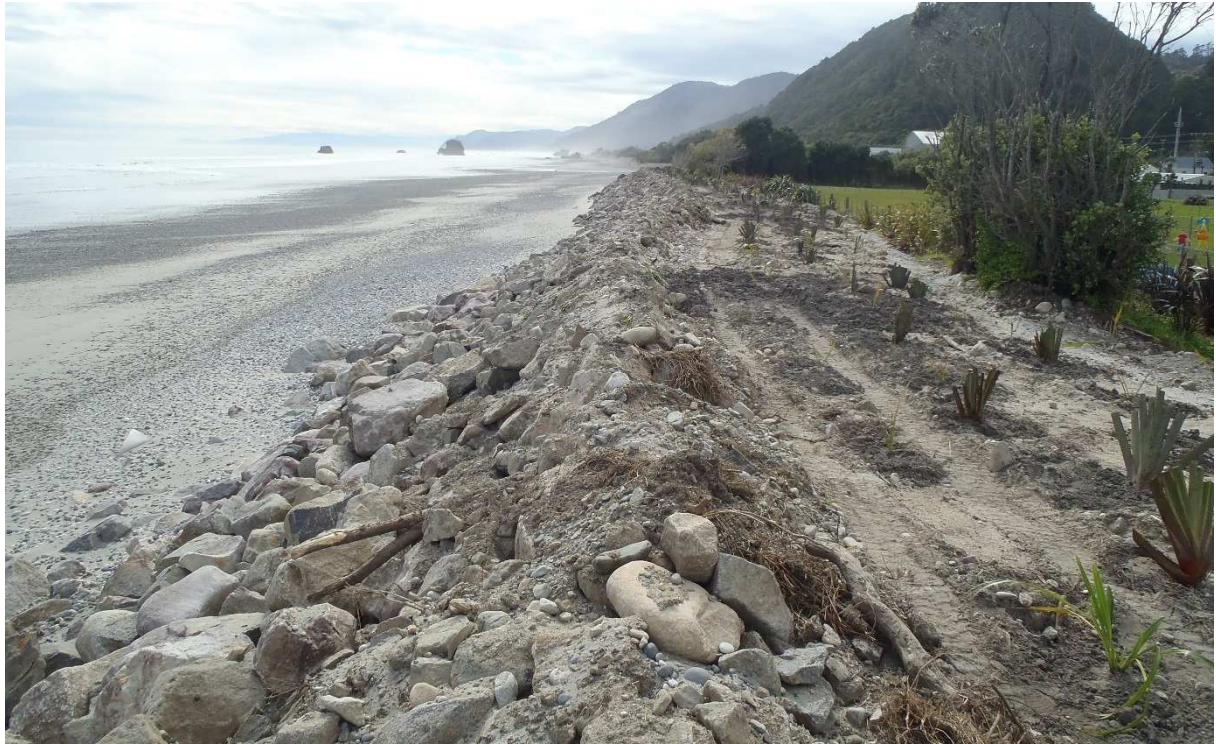
Figure 3-3: Recently constructed revetment at Granity school. Photograph looking north along-beach towards Torea Rocks (foreshore at upper left) from on top of revetment. [22 September 2015].
