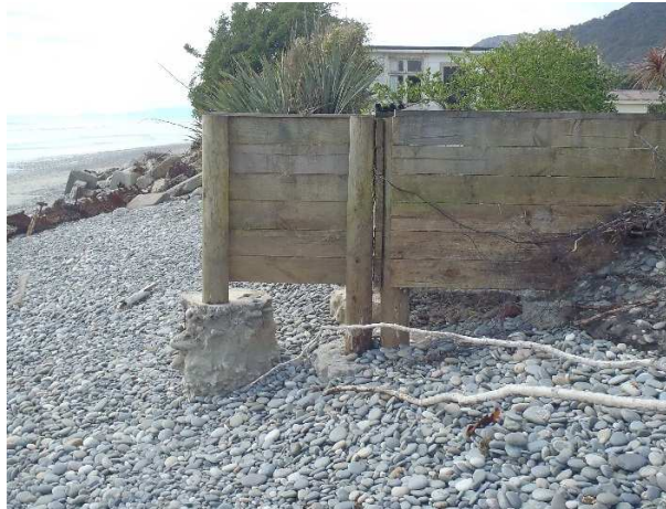
Figure 3-9: Erosion on northern side of Morris Creek exit showing proximity of houses (top centre) with eroding defences and nearby ad-hoc rubble defences (centre left). Photograph looking north from Morris Creek mouth at 14 Main Rd Ngakawau. [22 September 2015].
