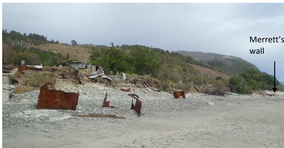
Figure 3-10: Ad-hoc rubble and steel defences along Ngakawau frontage between Morris Creek and 21 Main Rd. Photograph looking south east toward Morris Creek (annotation). [22 September 2015].
