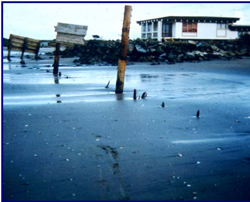
Figure 22: Erosion at Omaha North Spit subdivision after a severe storm in July 1978. The remains of a timber seawall can be seen. The wall was originally constructed along 1 km of beach to protect the subdivision. The dune system was levelled to provide better access and views to the beach. Following the erosion, the sand spit and tidal entrance to Whangateau Harbour were stabilised by several rock groynes built between 1979–1981, after an Act of Parliament was passed for emergency remedial work. [Photo: TM Hume]
