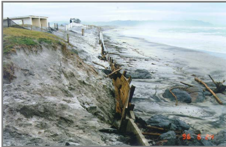
Figure 16: Re-emergence and destruction of a timber seawall at Bowentown (Katikati) during storms in 1996. The retaining wall was originally built some 20 years earlier to protect the shoreline from further erosion after storms in 1978. Subsequently the beach experienced an accretion cycle that built out the shoreline by 20 m and covered the wall by up to a 4 m depth of sand. [Photo (1996): RK Smith]
