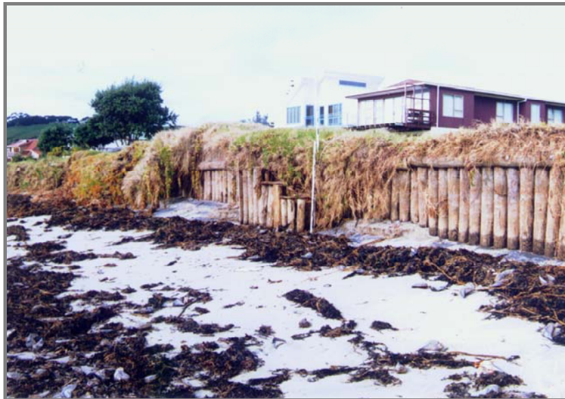
Figure 1: Timber seawalls have been placed to mitigate coastal erosion at Cooks Beach (Coromandel Peninsula). The photo captures the concept of “coastal squeeze”, where dwellings are quite close to an eroding beach, leaving little room for natural cycles of cut-back and advance of the shoreline. [Photo (1996): RK Smith]
