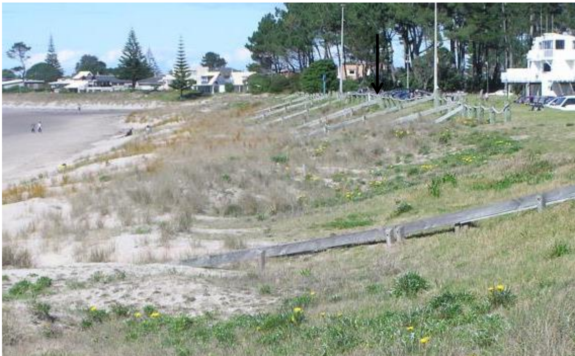
Figure 5: View of the south end of Esplanade Drive in August 2009 after a sustained period of dune building lasting several years (Photo: J Dahm). The 1978 erosion extended up to 2-3 m landward of the rope and bollard fence evident on the landward side of the dune.
