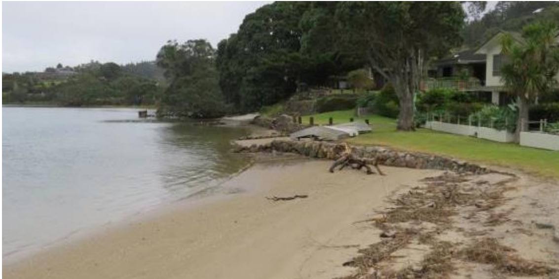
Figure 22: Shoreline at eastern end of Petley Parade. Note that the boundary of the public reserve is approximately where the white fence is in the foreground. The old block seawall was privately constructed, but lies on council reserve land.
