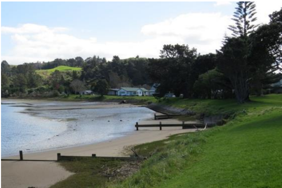
Figure 30: Shoreline protection works in Otahu Estuary, east of Kotuku Street. The gabion basket wall in the background is beginning to deteriorate.
