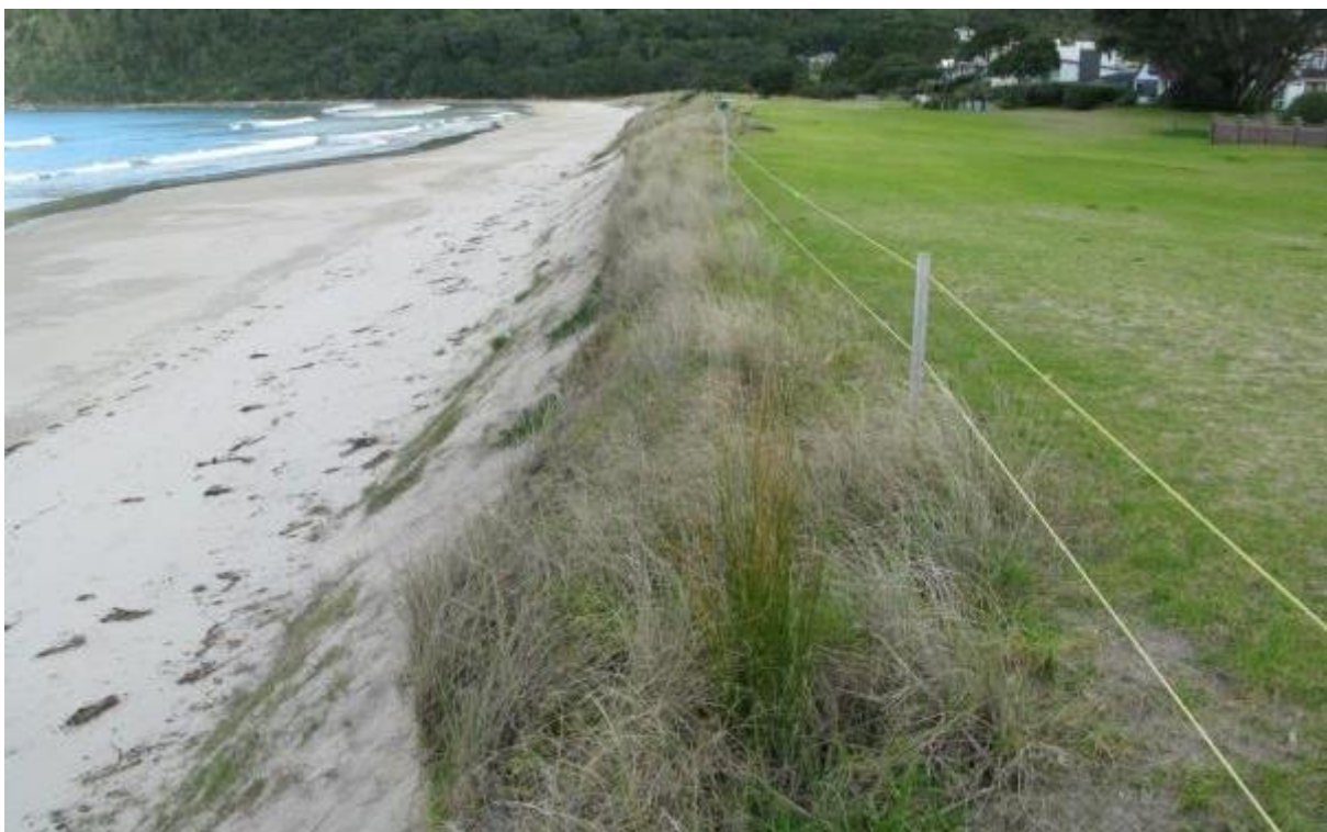
Figure 12: View of restoration area on southern Pauanui foreshore after period of dune erosion (in 2009 and following years). The narrow width of the restored native dune vegetation has largely been lost to erosion – with about 1m width remaining. This indicates the importance of having a natural dune of sufficient width to absorb the worst likely storm erosion. Otherwise, replanting has to occur after the erosion before natural dune repair can commence.
