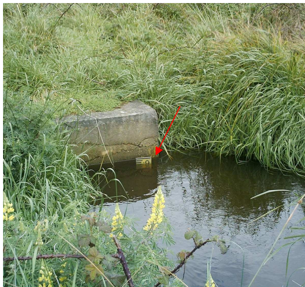
Figure 4.7 Site 3. The staff gauge (with miniTROLL attached) was located at a concrete culvert on Ngarara Stream where it enters the wetland system.
