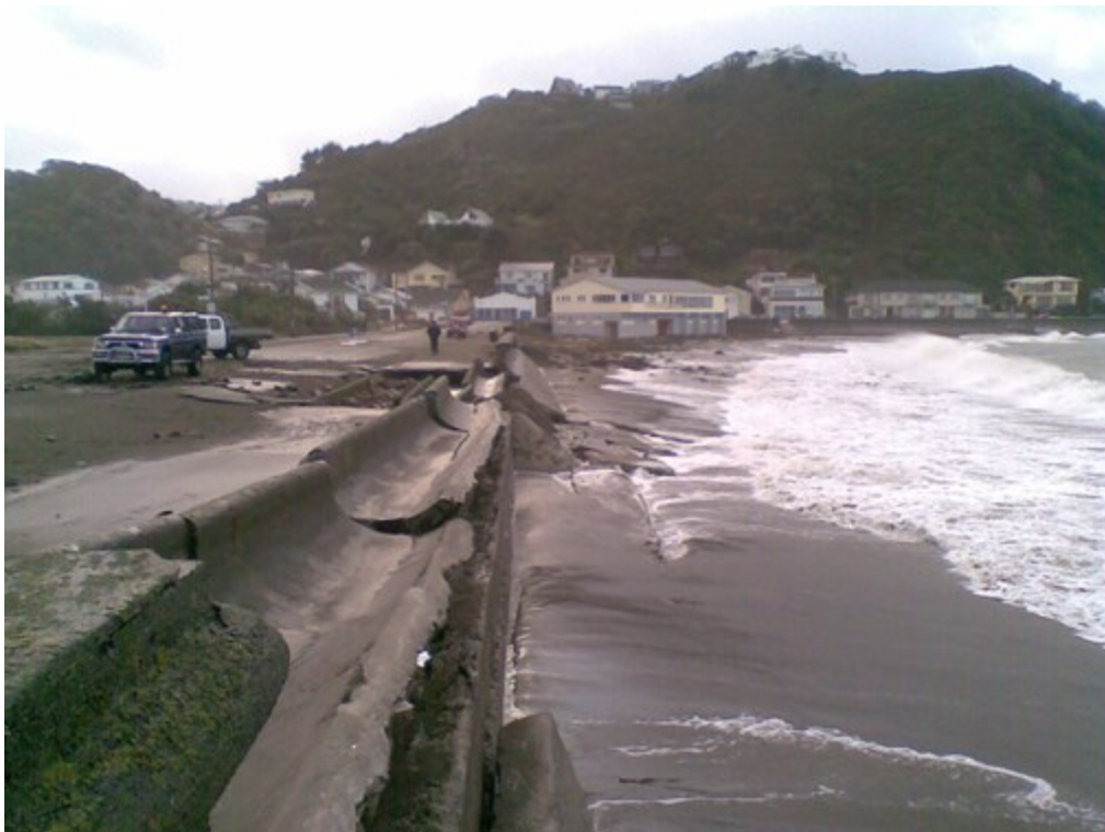
Figure 2 Damage to the Island Bay seawall following the June 2013 Storm Event (image: WCC)
