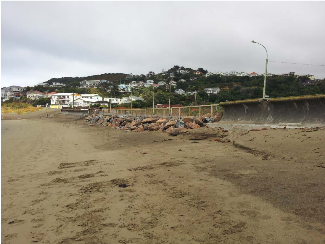
A-4 Failed section of seawall with temporary rock repair
