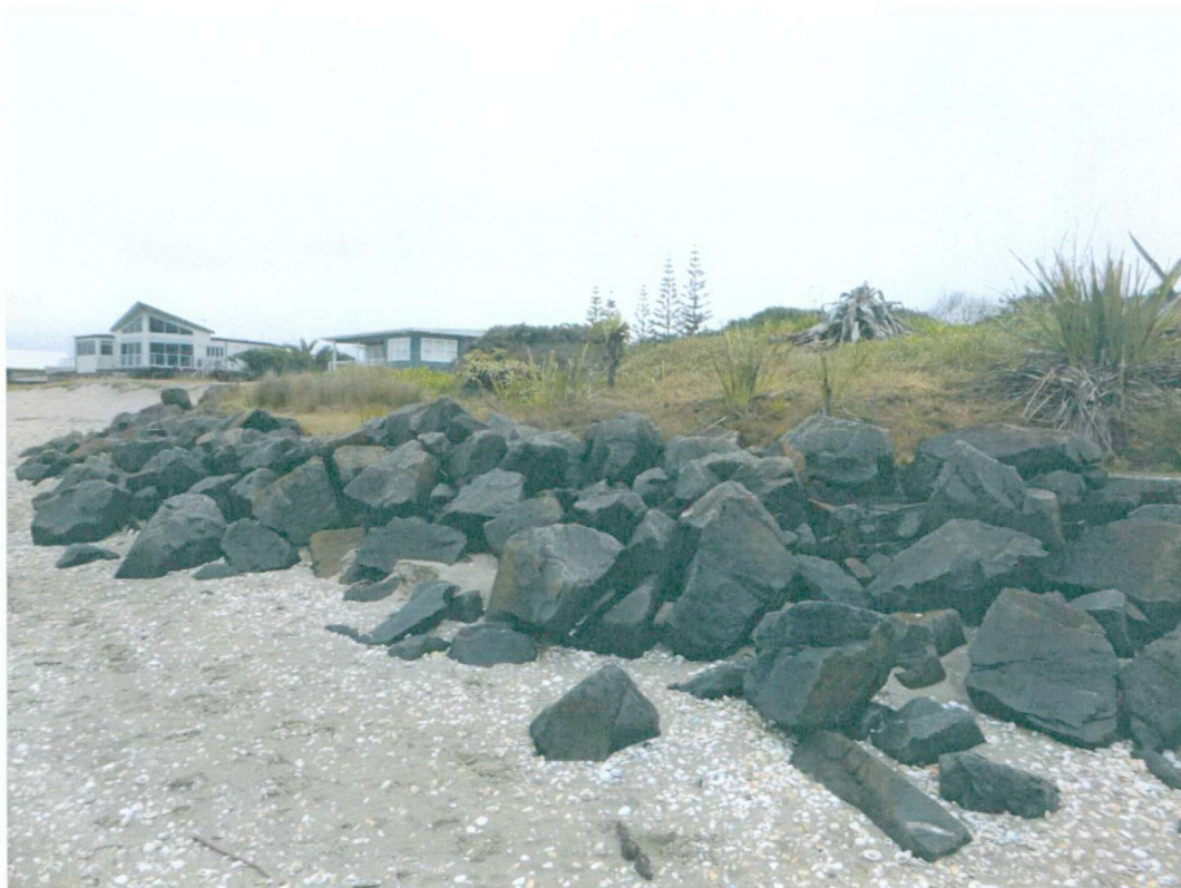
Photo 6: Southern extent of existing structure – showing landward retreat for unprotected area
