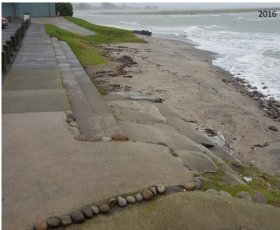
Figure 1.2: The access structure, carpark, GSC and surf club in 2014 and 2016. The area where erosion has been identified by the Community Board is visible at the toe of the access structure in 2014 (see red circle). Source: WBOPDC 2016.
