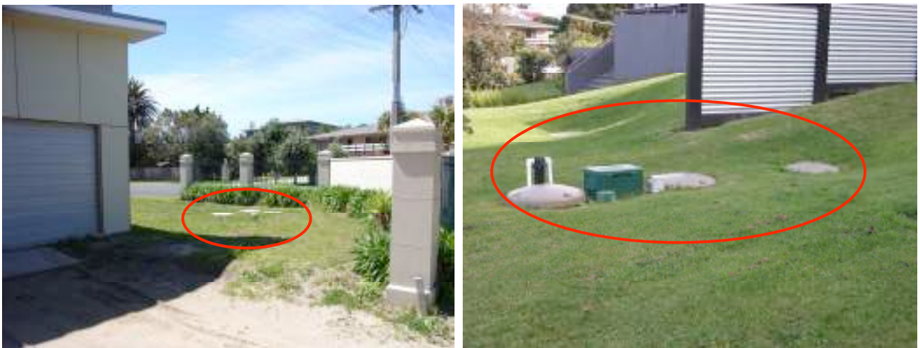
Figure 8 Two examples of the placement of on-site wastewater treatment systems in new developments (circled in red) and their location close to property boundaries, and with drainage field close to public footpaths and roads.
