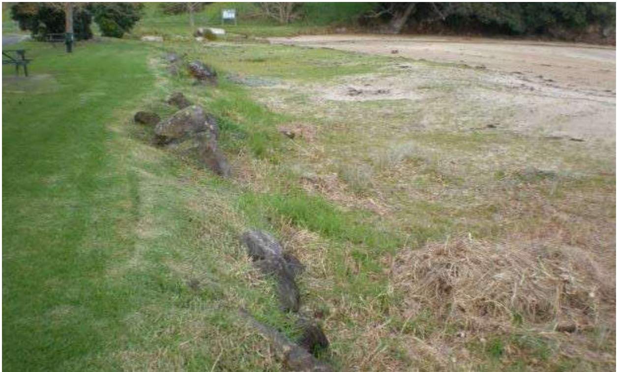
Figure 12: View of reserve frontage at eastern end of the beach showing rock protection placed to limit landward extent of stream and storm erosion. Note the low dune seaward of the rock wall.
