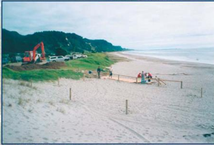
July 1998 Community members installing timber access for 4WD vehicles. Excavator is creating a bund to direct vehicles onto the access. Planting started after the fence was completed.
