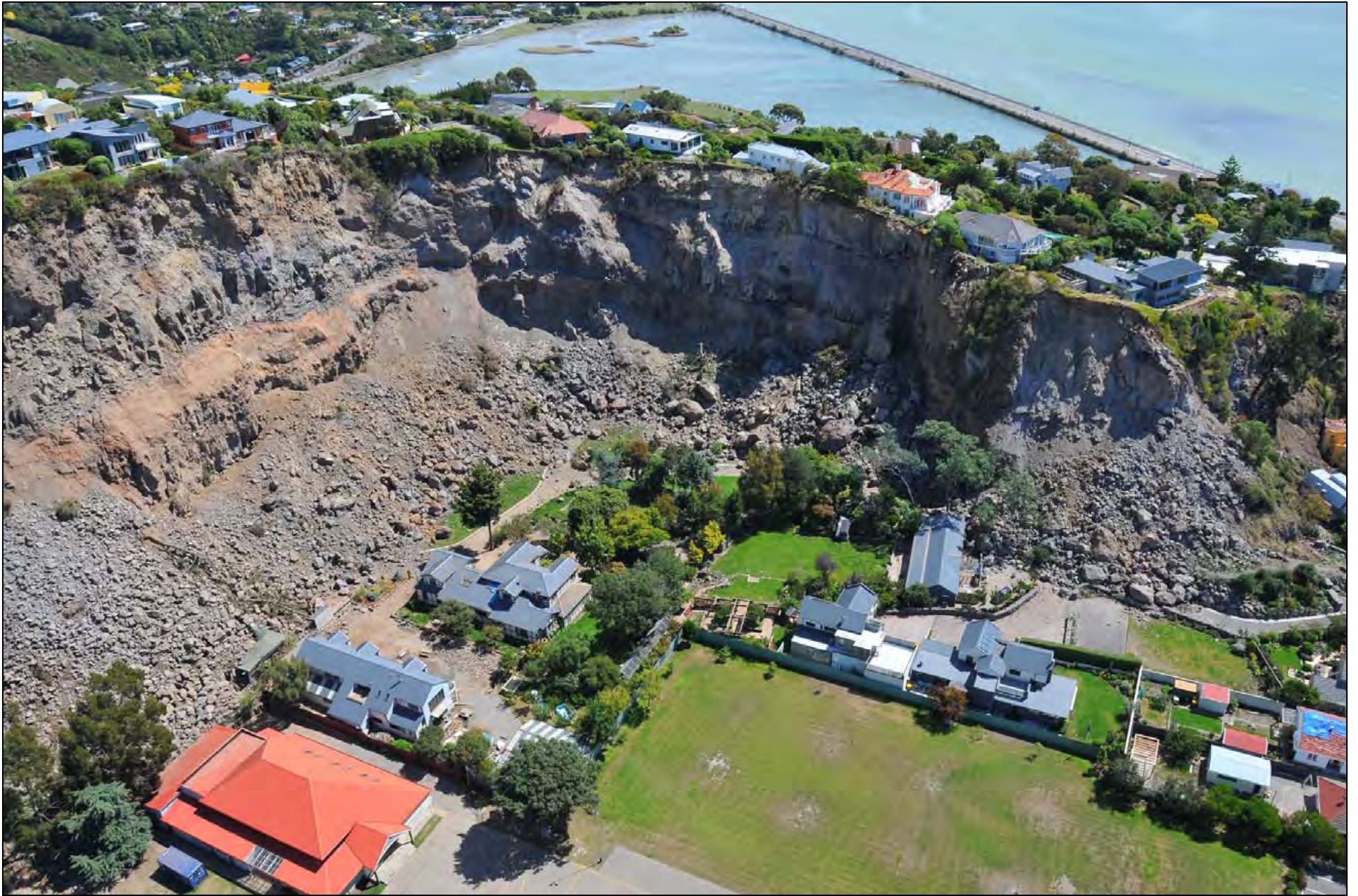
Photo 19. Large rock falls on the cliff behind Redcliffs School and Moa Cave Guest House, Redcliffs ( GNS Photo-GTH_5792 ).
