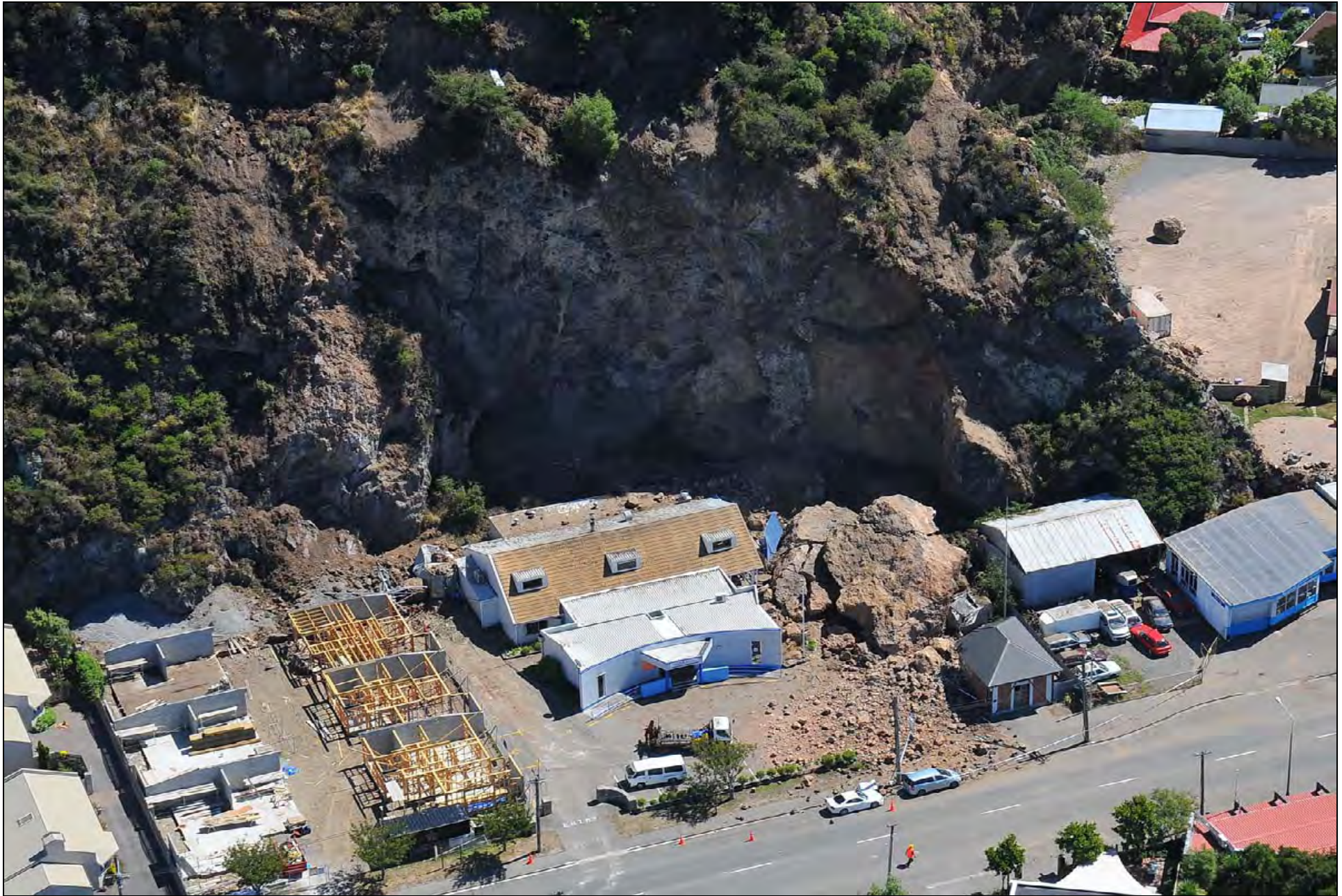
Photo 6. Large rock fall behind the RSA Building at 34 in Wakefield Ave, Sumner (rock fall fatality reported at building site left) ( GNS Photo-GTH_5708 ).
