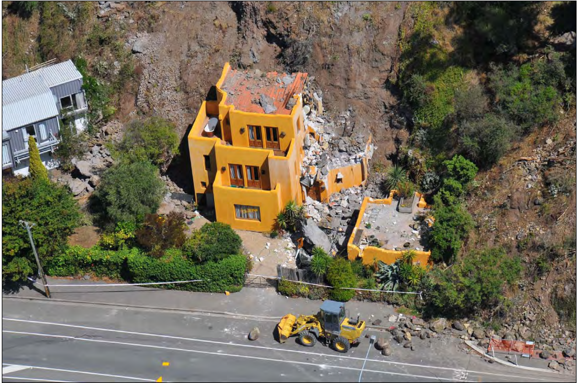
Photo 25. Rock fall on to house at 116A Main Road, Redcliffs ( GNS Photo-GTH_5823 ).
