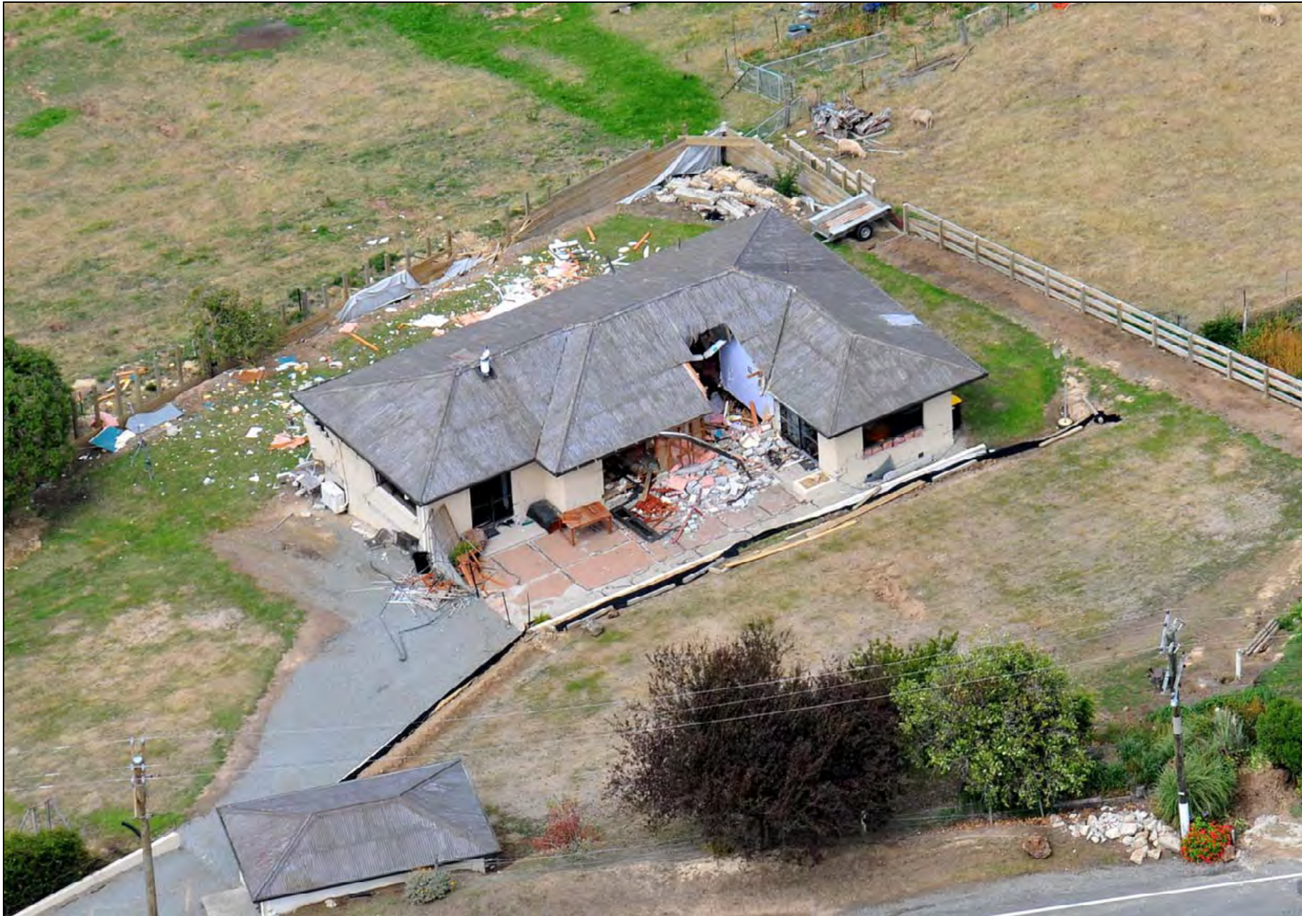
Photo 26. House at 241 Governors Bay Road, Rapaki, hit by a large (~3 m long) boulder 3 km west of Lyttleton ( GNS Photo-GTH_5842 ).
