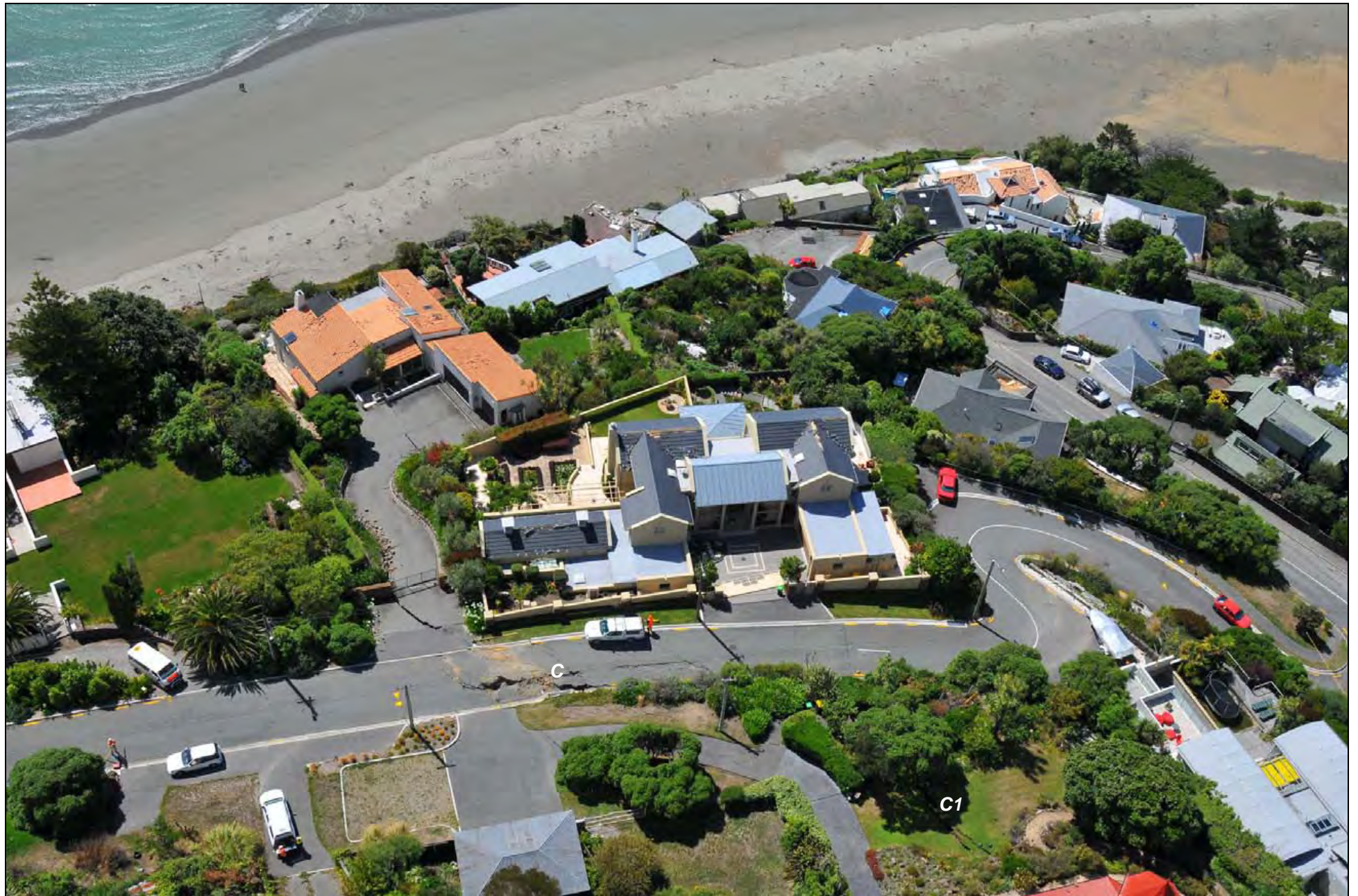
Photo 14. Cliff top cracking (C) along the cliff edge and affecting houses (C1) in Kinsey Terrace on Moncks Bay headland (GNS Photo-GTH_5771).
