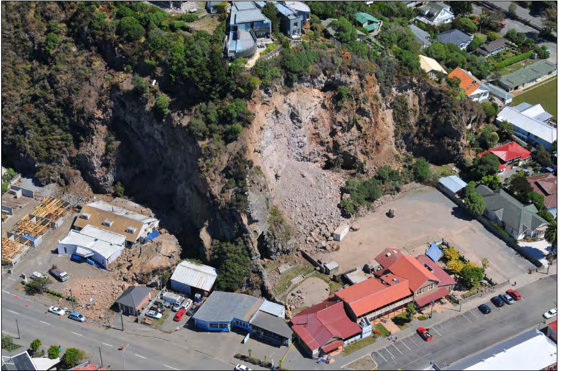
Photo 7. Rock falls on cliff face behind RSA and Backpackers buildings at corner of Wakefield Ave (left) and Nayland Street (right), Sumner ( GNS Photo-GTH_5712 ).
