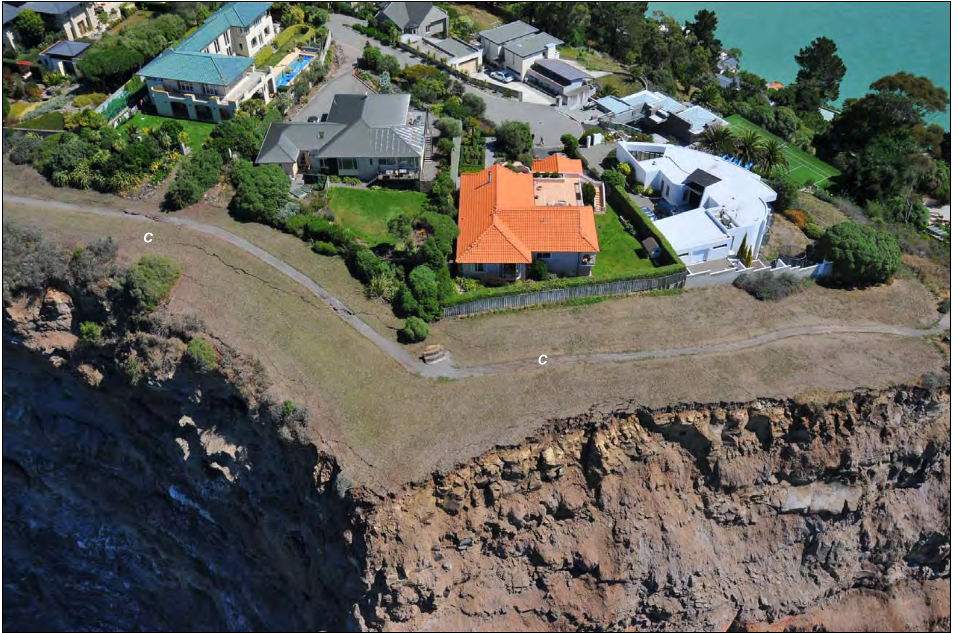
Photo 3. Tension cracks (C) along the cliff edge close to houses on Searidge Lane at Sumner Head (GNS Photo-GTH_5661).
