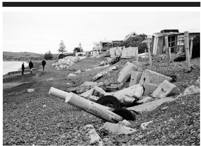
Figure 9. Erosion at South Haumoana threatening several homes, with the failure of their shore-protection structures (2001 photo).
