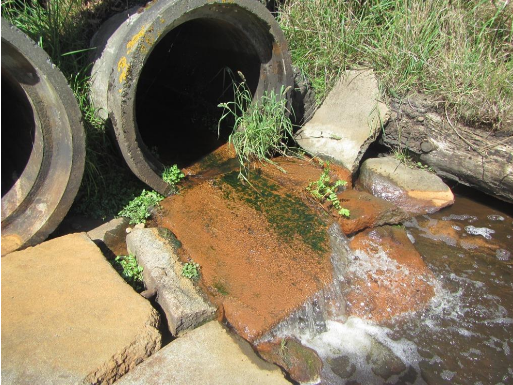
Plate 11: Culvert pipe being a partial impediment to fish passage in the channel downstream of the Pukepuke Conservation Area. 15 March 2017.
